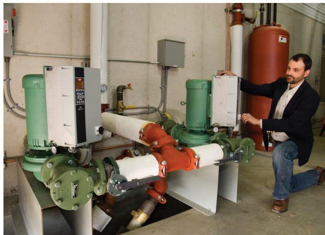
Matt Aungst, who designed the distribution portion of the project tests redundancy of the two pumps that serve the entire project. Pump A runs as "duty," leaving pump B for backup. After 84 hours of run-time, the pumps automatically switch roles. (Photo courtesy of Total Energy Solutions)
