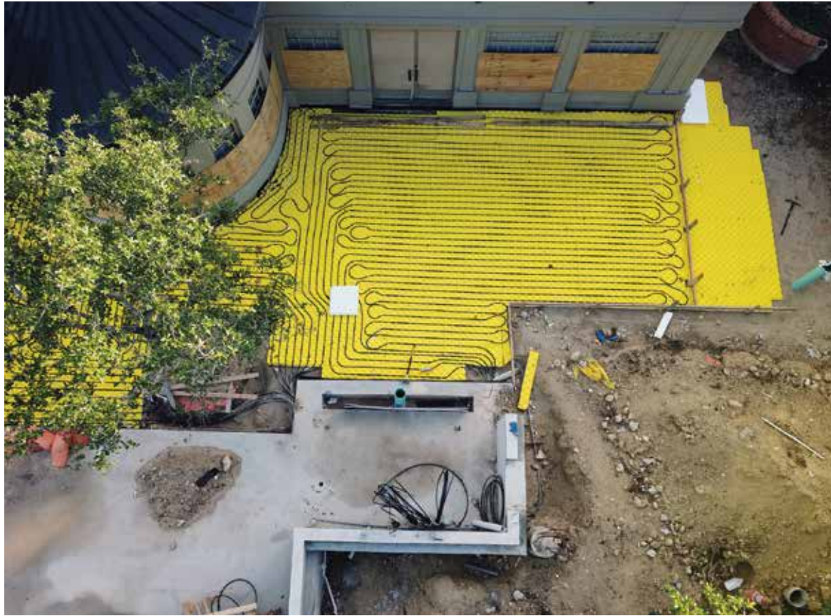
GROWING ACCEPTANCE: Jim Erhardt, hydronic product specialist, Watts, hopes to see a growing acceptance and understanding of radiant cooling systems and the role they can play in building occupant comfort and system operating efficiency.
