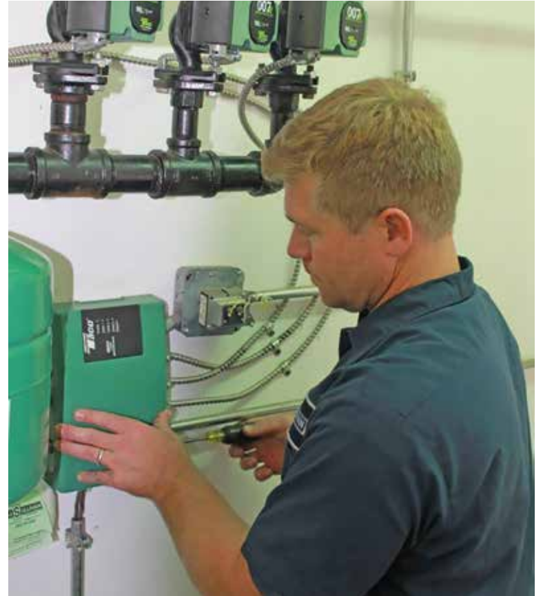
IMPROVED INSTALLATION: The past two decades have seen seismic change in the circulator and pumps industry, with changes that have vastly improved things for installers.
