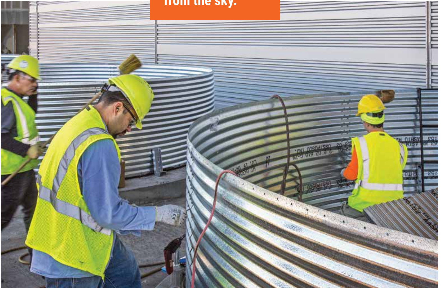
A new cruise ship terminal at Pier 27 in San Francisco, California, developed a rainwater harvesting system to recycle water in surrounding buildings.
