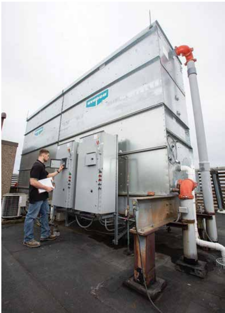
TWO TOWER: New Evapco cooling towers replaced the units that had served Wall Street Tower since it opened.
