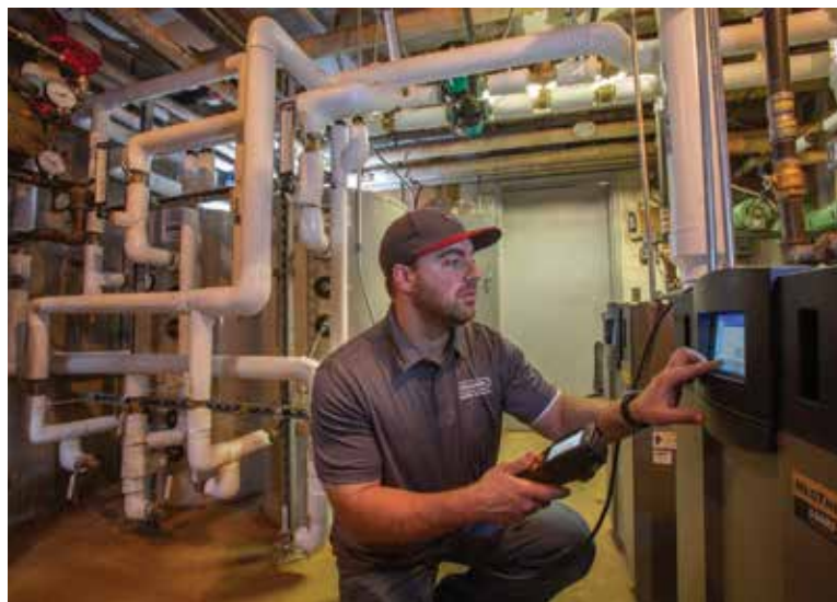
IMPRESSIVE CONTROLS: A tech with Denron Plumbing and HVAC LLC checks the controls on a Laars boiler.
