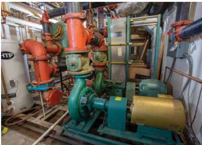
KEEPING WARM: The updated heating system keeps tenants warm during the chilly winters of New England.
