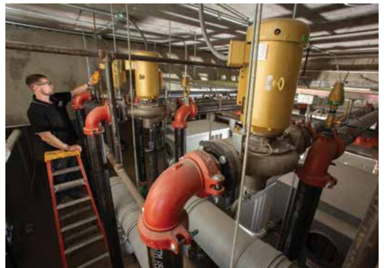
BIG JOB, SMALL DETAILS: A technician ensures that the mechanical system is in working order.
