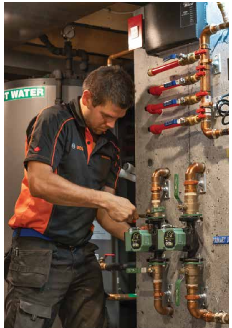
CRAFTSMANSHIP MASTERY: Orest Omeliukh, founder of Blackrock HVAC Ltd., builds the Bentley of HVAC systems as a craftsman and designer.
