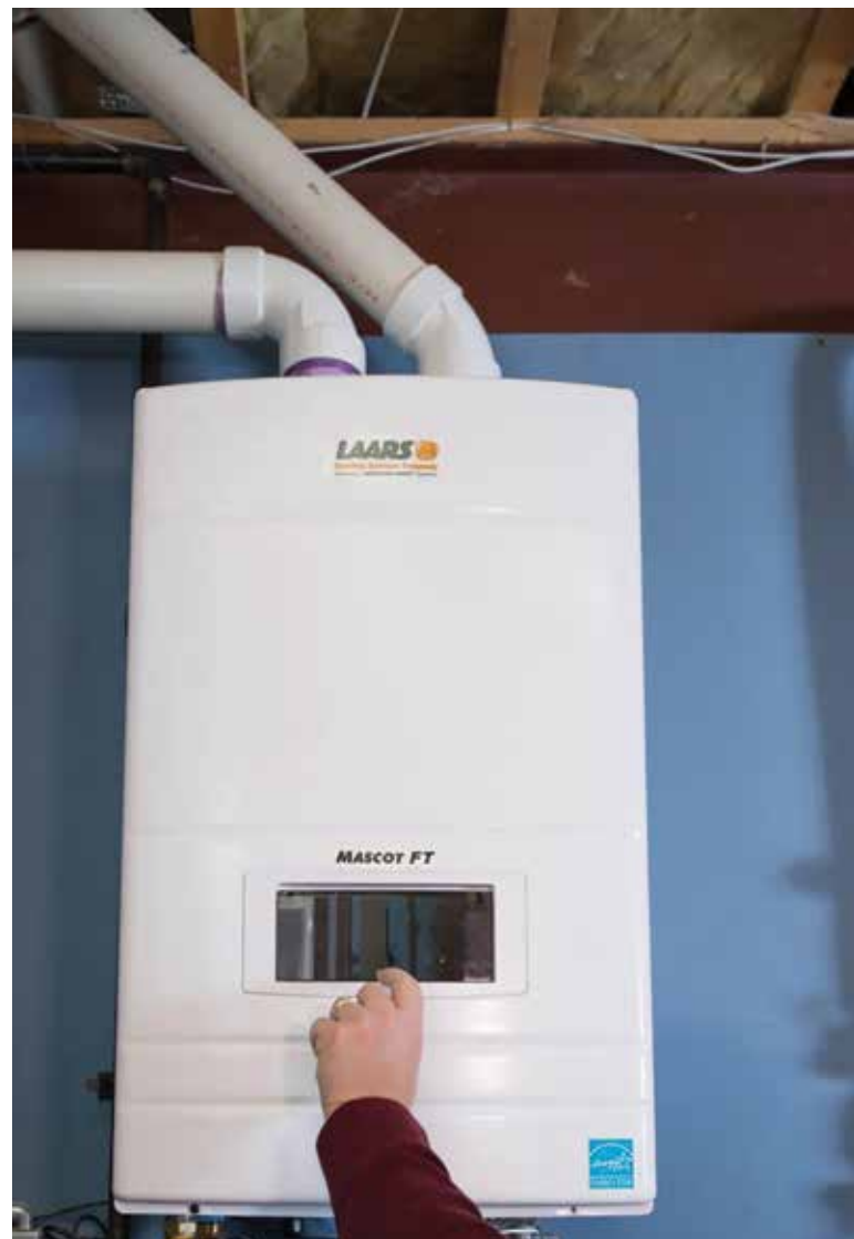
KNOW WHAT WORKS: A Laars Mascot FT boiler was chosen to replace the original Laars heat plant because it had worked so well in the past.
