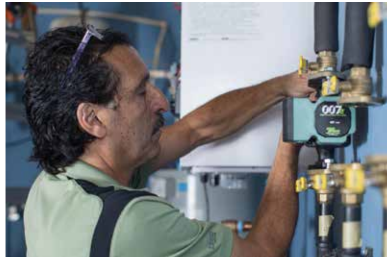
RATE OF FLOW: By reducing flow, variable-speed ECM circulators increase system delta T, so the system requires much less fuel to run.
