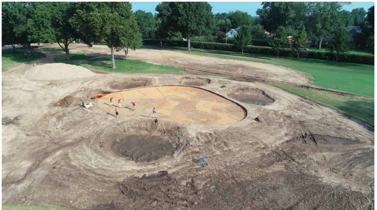
BIG JOB: After the country club voted to install green conditioning systems in 2016, the 300-acre property was closed in early 2018 to permit renovations.
