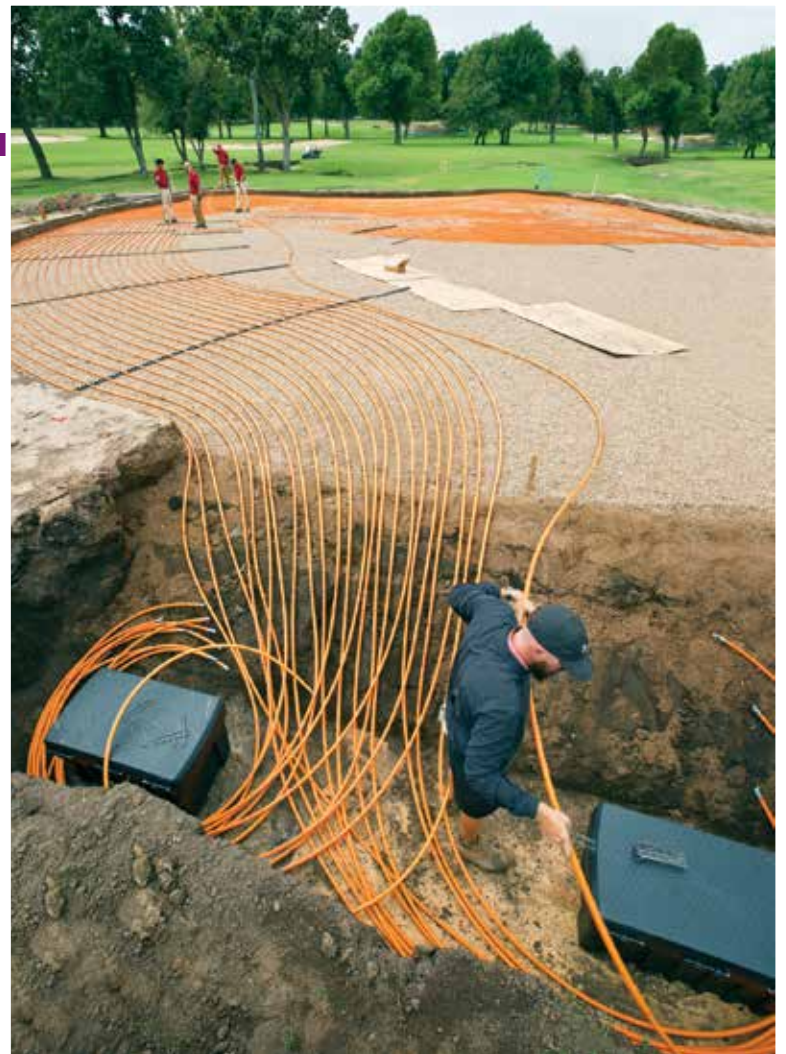
DOWN TO IT: All radiant loops terminate in an underground manifold box.
