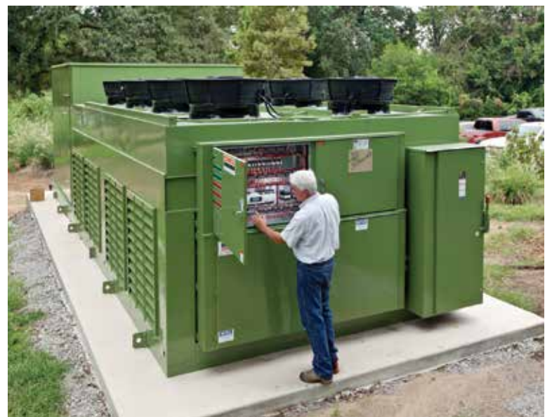
ONCE OVER: Cary Pestel, Boone & Boone Sales, looks over a large air-to-water heat pump installed at SHCC.
