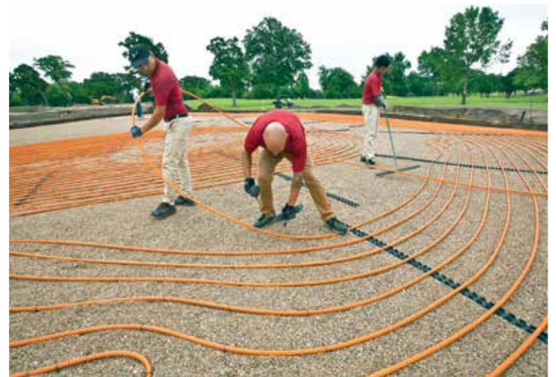
LAYING IT OUT: SHCC grounds crew members (left to right) Oscar Mendez, Matthew Jackson, and Edwin Gomez lay Watts RadiantPERT tubing on what will become a green surface.
