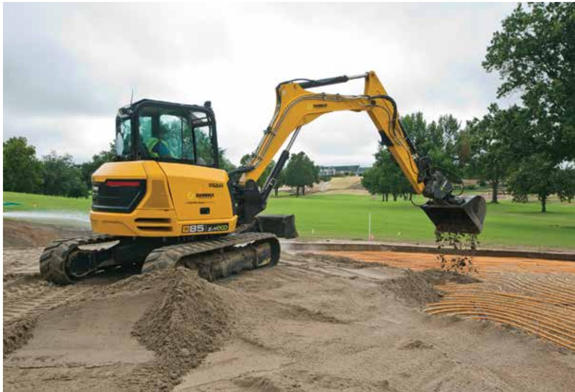
COVERING IT UP: Once tubing is installed, a layer of “greens mix” – made of sand and peat – is carefully distributed before the green is seeded.
