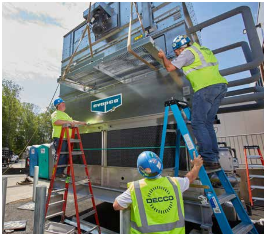
Decco riggers complete cooling tower installations at New England BioLab's new facility.
