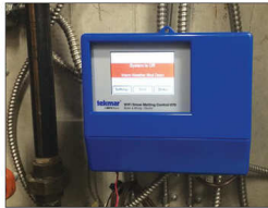
Above: A tekmar 670 snowmelt control simply remains inactive during the off-season but is ready for duty as winter approaches. Photo: Watts.
