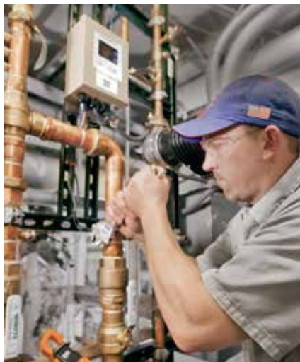
Ian Walters, project manager, Lexington Plumbing (left), and Jamie Shibel, outside sales for the manufacturer’s rep firm, Mack McClain and Associates, make adjustments to the mixing valve’s setpoint.
