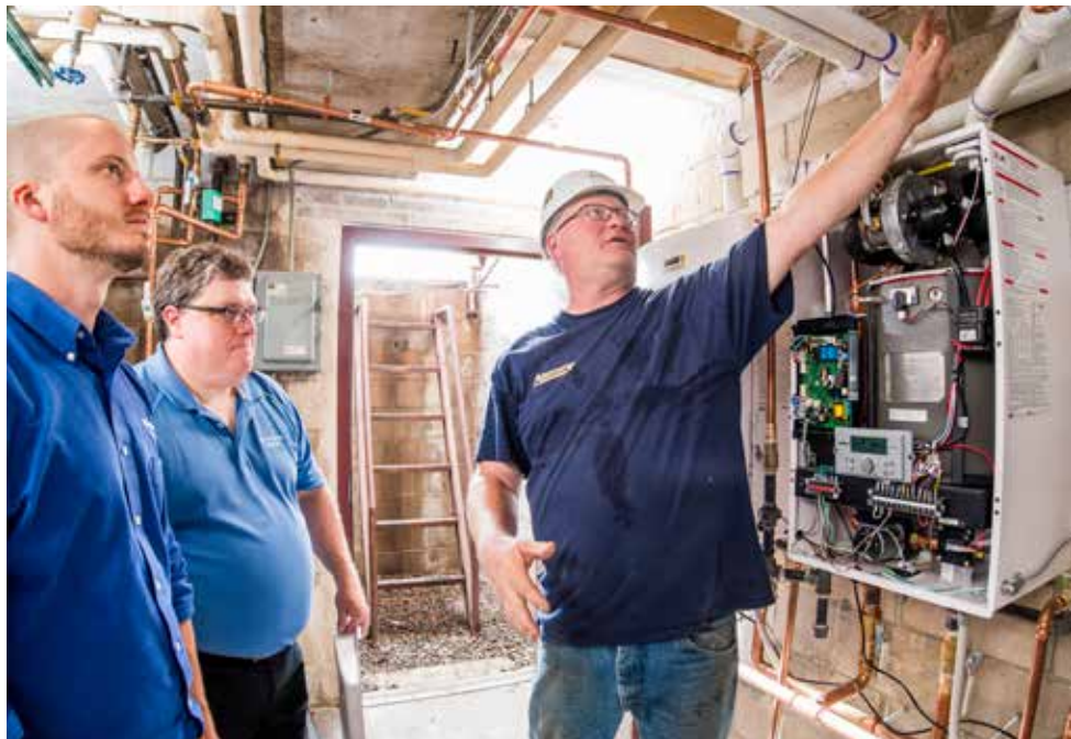
ANALYZE THIS: Kruse (left) completes a combustion analysis on one of the Laars Mascot boilers. Working with him are Larry Sandberg (middle), field support and technical trainer, Michel Sales, and Mike Jackson (right), Associated Mechanical pipefitter foreman.
