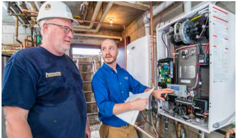
FINAL TOUCHES: Mike Jackson (left), pipefitter foreman, Associated Mechanical, and Nick Kruse (right), field support and trainer, Michel Sales, perform final boiler commissioning in one of the mechanical rooms.
