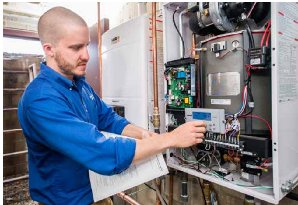
HEAT CURVE: Kruse sets up a heat curve for one of the Laars boilers. With an efficiency of 95 percent AFUE, input of 199 MBH, 10:1 turndown, and the capability of cascading up to 20 boilers for larger structures and redundancy, the new boilers have given managers and residents peace of mind.
