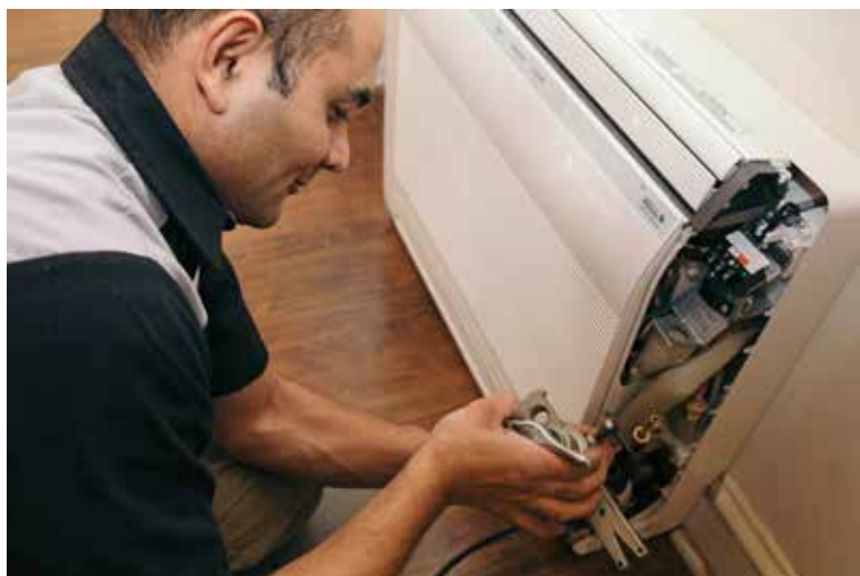
FLOORED: Man Khadka, installer, Vertex Mechanical Inc., installs a floor console unit in the main fellowship hall.
