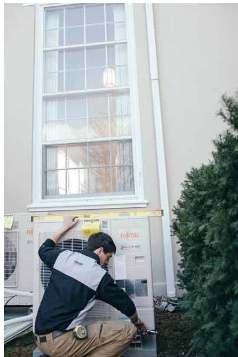
WINTER READY: Jared Fox, lead installer, Vertex Mechanical Inc., fastens snow legs to a Fujitsu Halcyon multizone condenser outside the Lititz Moravian fellowship hall.
