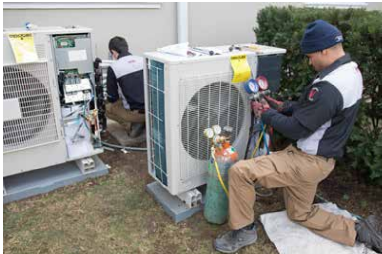
CHARGED UP: Lester Gonzalez (foreground), installer, Vertex Mechanical Inc., charges a Halcyon unit while Jared Fox (background), lead installer, organizes refrigerant line sets for units serving the fellowship hall.
