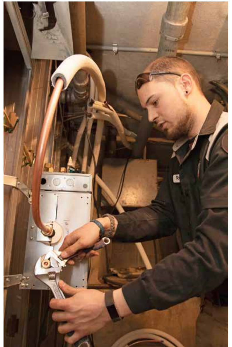
BRANCHING OUT: Ryan Schweitzer, installer, Vertex, works on a Fujitsu branch box in a mechanical area in the basement of the fellowship hall.
