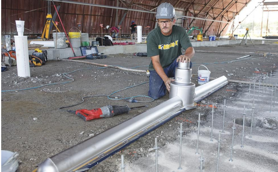
Denny Peace, an A.L. Miller plumber, inspects an upside-down, below-grade section of Blücher HygienicPro trench drain prior to installation. The drain sections come completely assembled.
