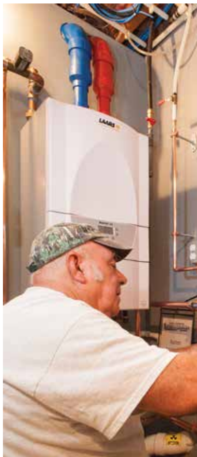
INSTALLATION COMPLETE: Dan Williams, installer, Haldeman Mechanical, completes the installation of a Watts expansion tank.
