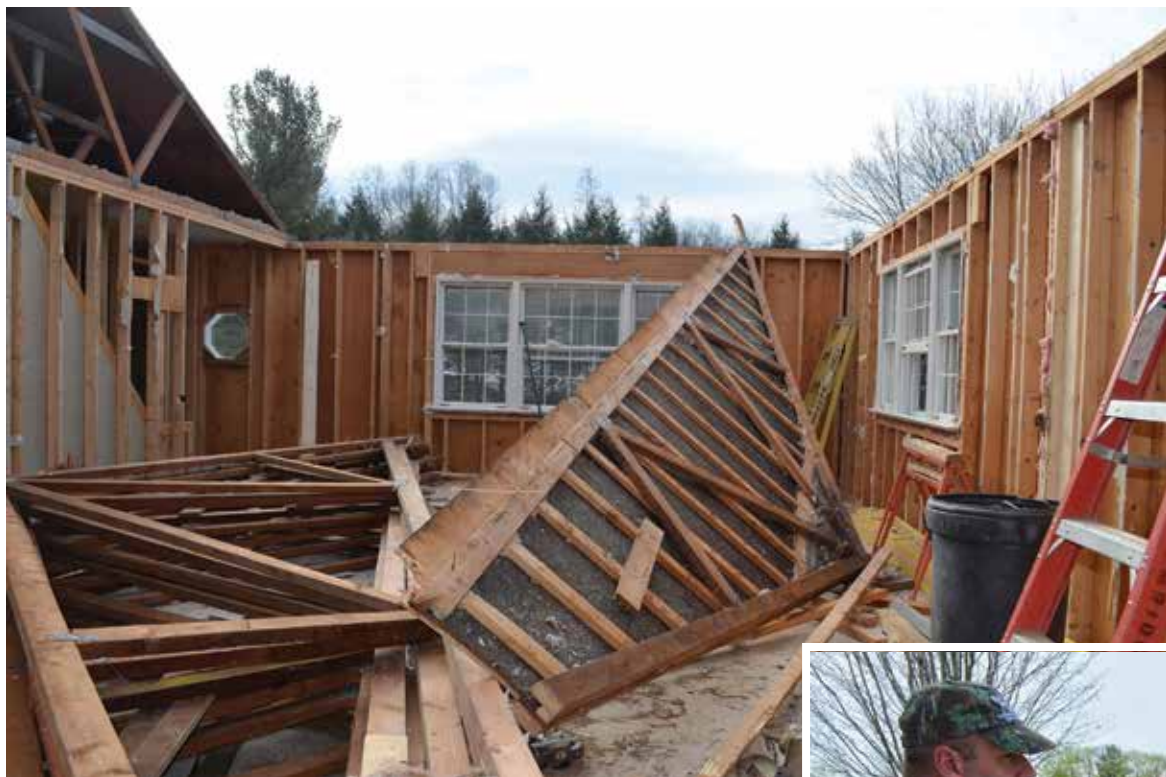
EXTREME MAKEOVER: During the remodel, most of the home's roof and all of its windows, doors, and electrical and mechanical systems had to go.
