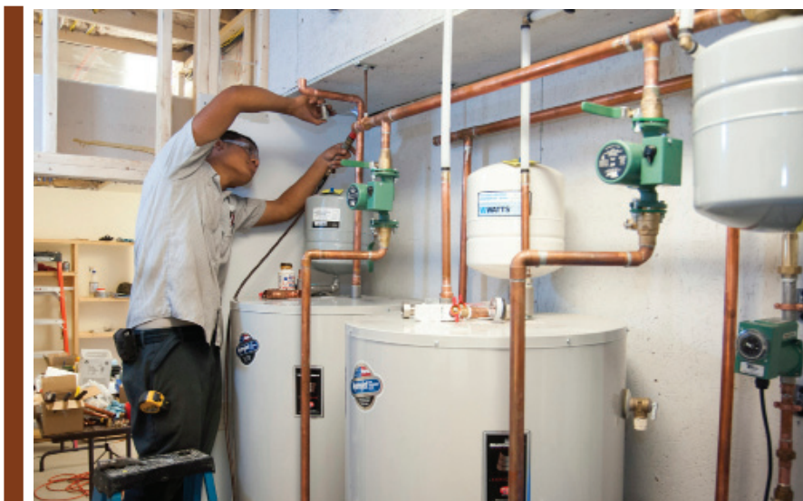
120-gallon Bradford White tanks and Taco circulators
