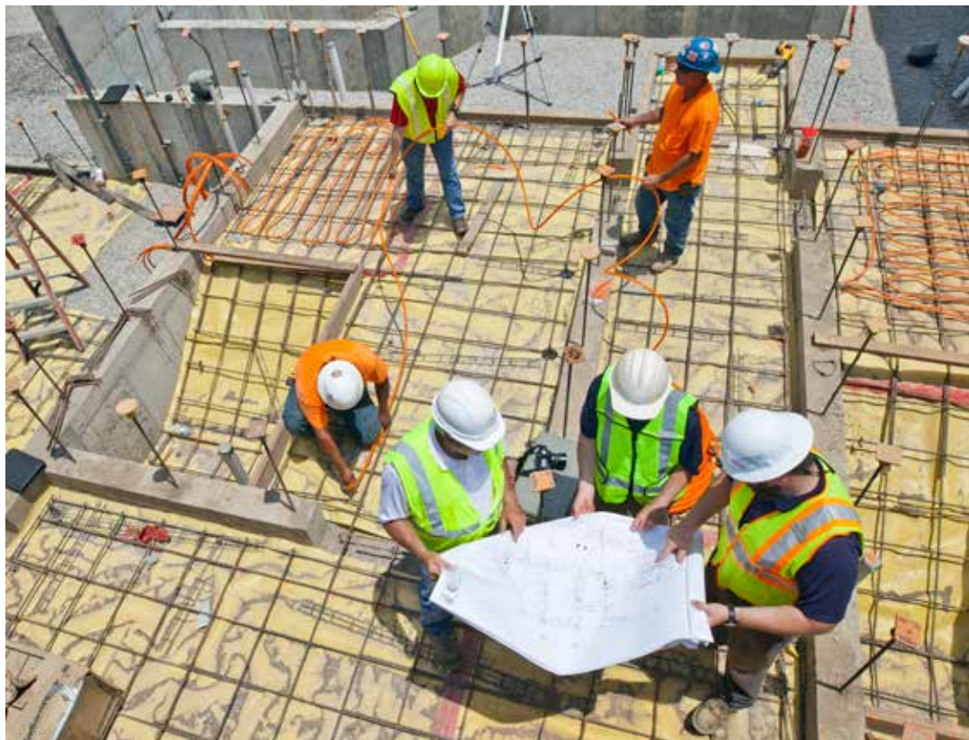
Cary Pestel, owner of Tulsa-based Boone & Boone (left, foreground) reviews radiant heat layout with engineers during installation of Watts RadiantPEX+ for an interior animal space within the Lost Kingdom exhibit prior to the concrete pour.
