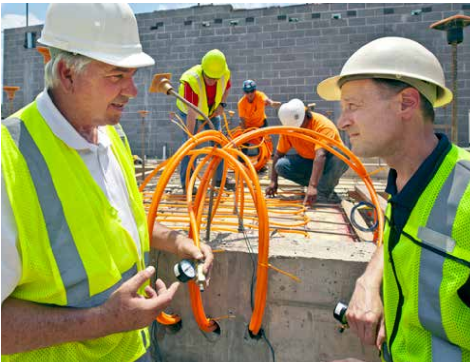
Cary Pestel, owner of Tulsa-based Boone & Boone (left), and Greg Sutcliffe, engineer at Tulsa-based Phillips + Gomez (right), discuss radiant system pressure during installation of Watts RadiantPEX+ for an interior hydronic radiant space.
