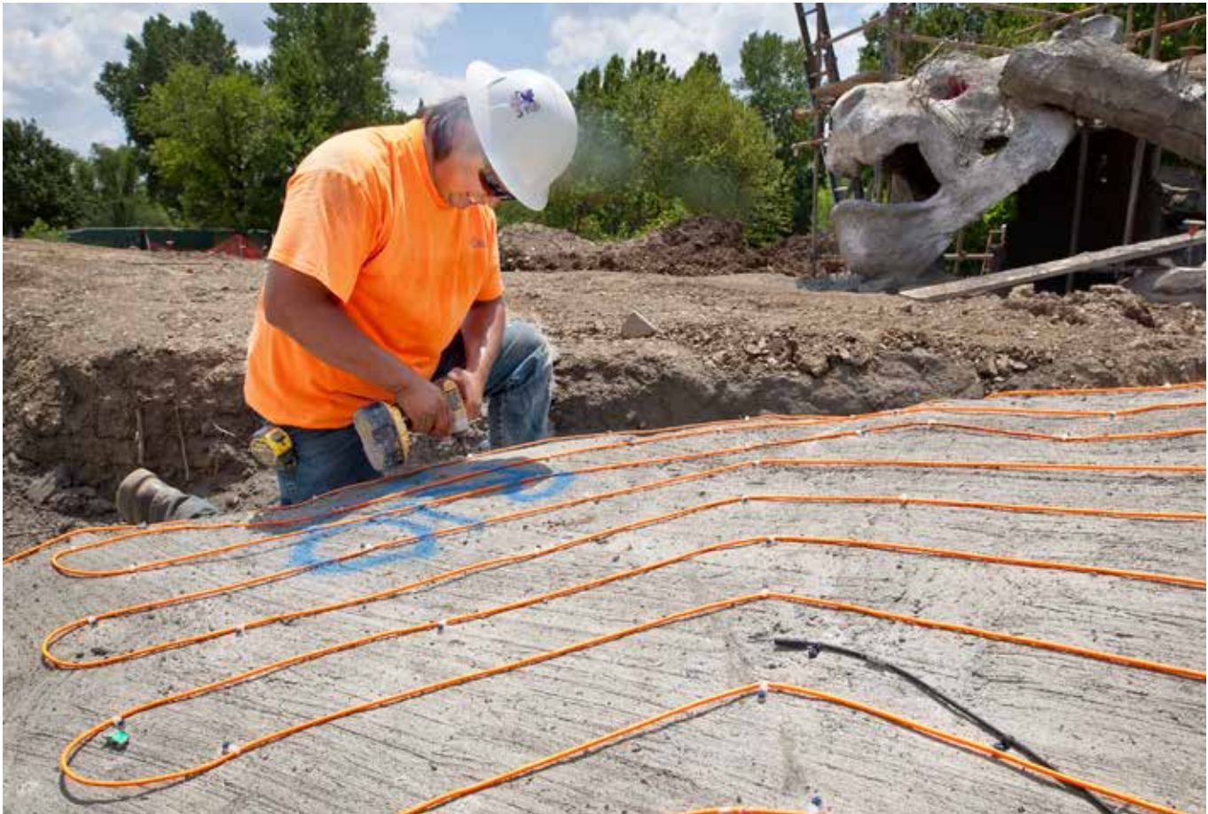
Johnson Tiger, McIntosh, works to install the more than 50 lineal ft. of ProMelt electric radiant heat cable encased in each of the 24 sq. ft. tanning beds, dishing out 50 watts per sq. ft. The hot rocks will be located strategically to provide optimal viewing for guests and offering animals the chance to seek warmth whenever they like.
