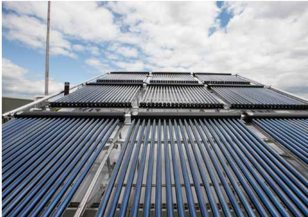
Consider additional storage needs early when designing a commercial solar thermal system because the cost for larger storage is best during installation.
