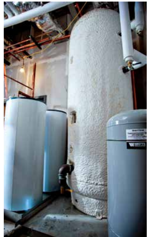
The Marine 9 firehouse has a 475-gal. Niles Steel Tank installed where glycol lines run from the solar thermal arrays to the heavily-insulated tank.
