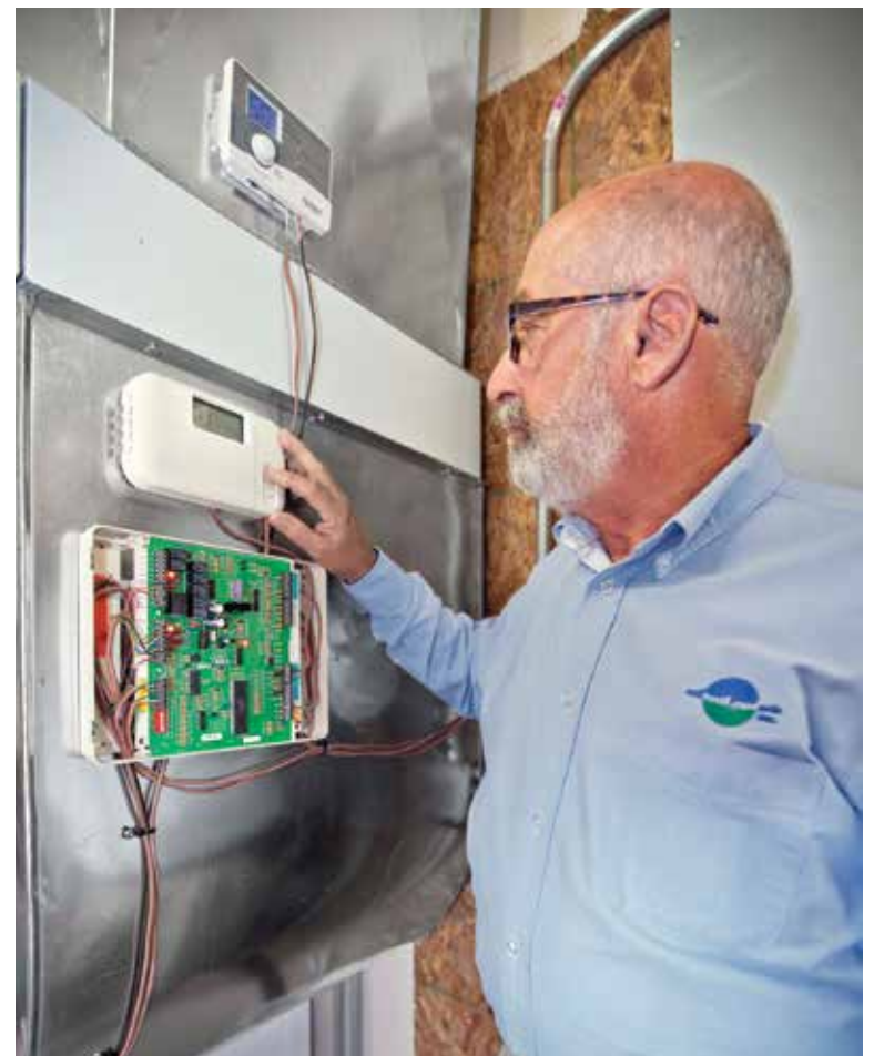
CONTROLLED CLIMATE: Dick Burhans, president of ReBearth Products Inc., checks the building's set point temperature.
