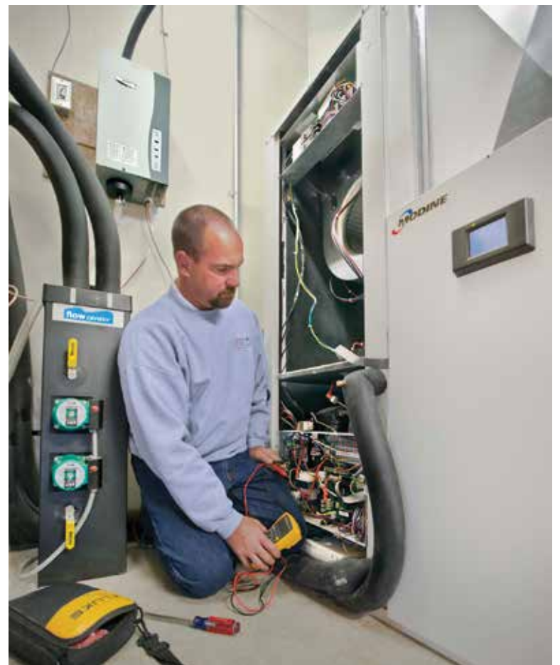
ENHANCED EFFICIENCY: Anthony Sherman, owner of Sherman Co. LLC in Adel, Iowa, checks a 5.5-ton Modine Geothermal unit; one of two similar units at the museum.
