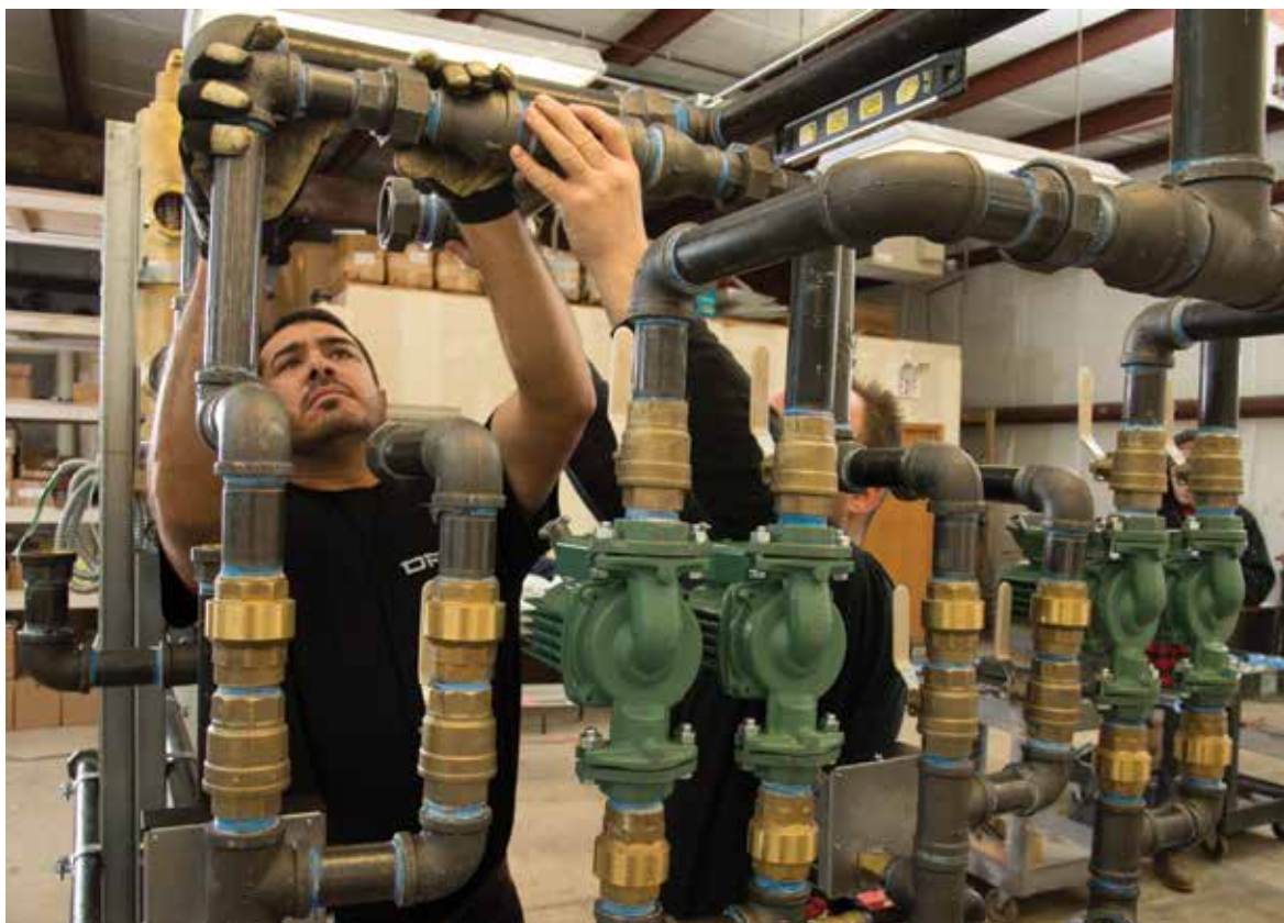
PROPERLY POSITIONED: Taco circulators are lined up during preassembly of near-boiler piping performed by the hydronics professionals at Romeoville, Illinois-based manufacturer's rep firm and custom manufacturer, Metropolitan Industries Inc. They prepared 19 fully assembled, split-skid boiler packages to reduce down time during installations at an apartment complex by Plainfield, Illinois-based plumbing and mechanical contracting firm DRF Trusted Property Solutions.
