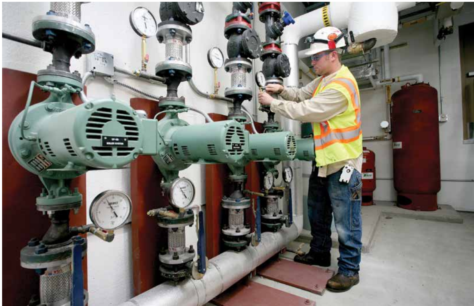
PUMPS AND PEDESTALS: Steve Bothell, Weldin's lead foreman, attaches a pump pressure gauge to one of the main Taco LoadMatch pumps for the two 3-inch primary mains at this Professional Military Education Center. The heavy-mounting pedestals allow floor support for the pumps, which is especially important in seismic regions.
