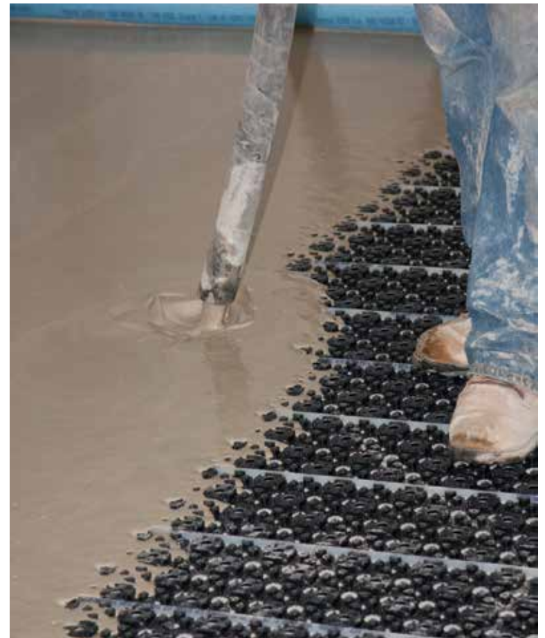
READY FOR RADIANT: A radiant installation with Fast Trak and Radiant Ready 30E takes place at the Perez Home, Minnesota.
