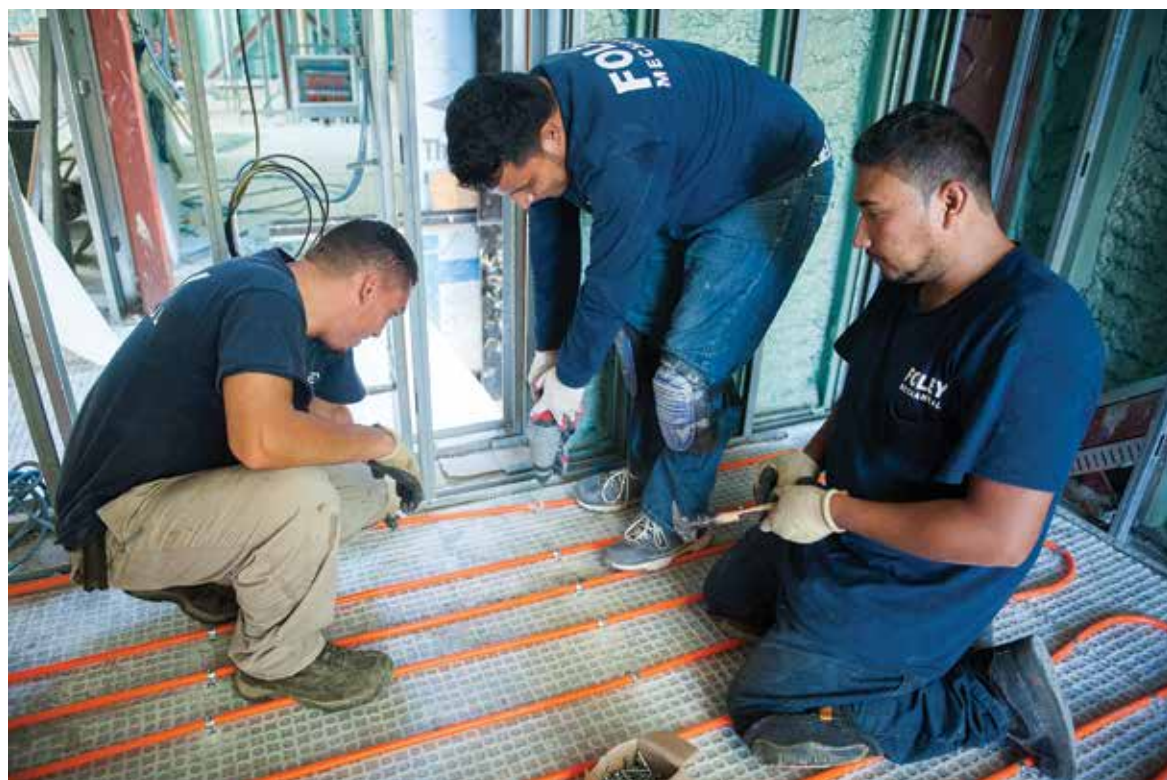
TUBING TRIO: Technicians for Foley Mechanical Inc. in Lorton, Virginia, secure Watts Radiant PEX tubing to the floor of a facility in Washington, District of Columbia.
