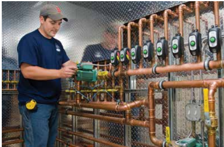
PERFECT PIPES: A technician with Woburn, Massachusetts-based Central Cooling & Heating Inc. completes a hydronic installation at a custom home near Boston. The variable Delta-T pump provides circulation for a multizone hydronic system served by Zone Sentry zone valves.
