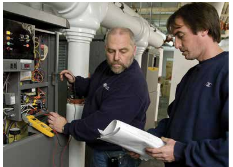
WORKING TOGETHER: Ike Beyer, owner of Islip, New York-based Integrated HVAC Systems and Services Inc., works with an employee during installation of Laars Rheos+ boilers at a retirement facility.
