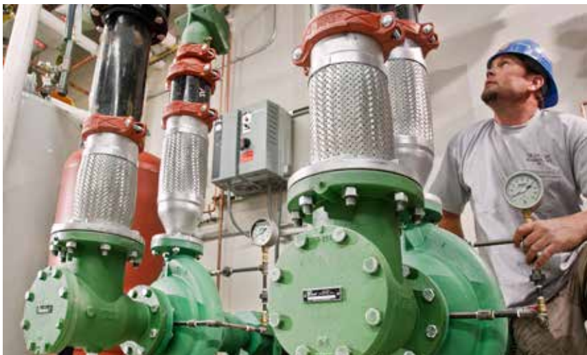
4G Project Foreman Hans Halverson works on one of four VFD-powered pumps that serve the oncology facility's heating and cooling systems.
