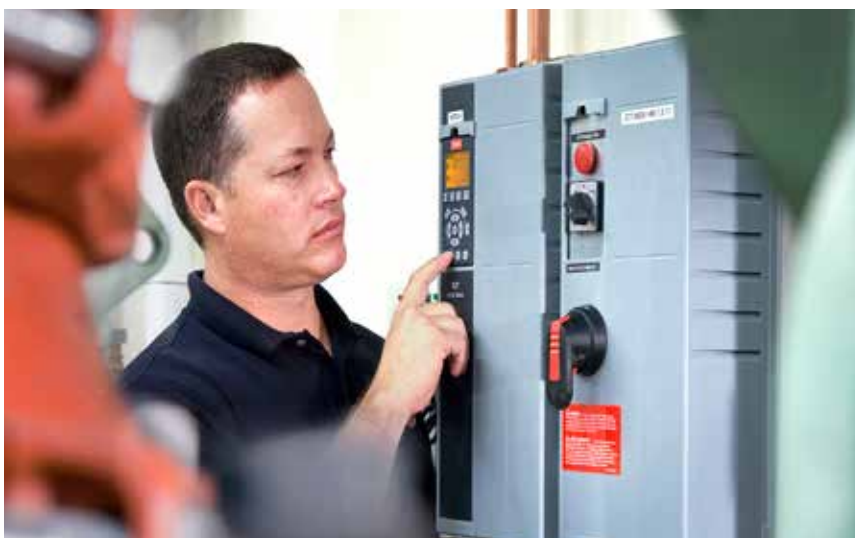
4G Project Manager, Cory Hanninen programs a VFD during commissioning.
