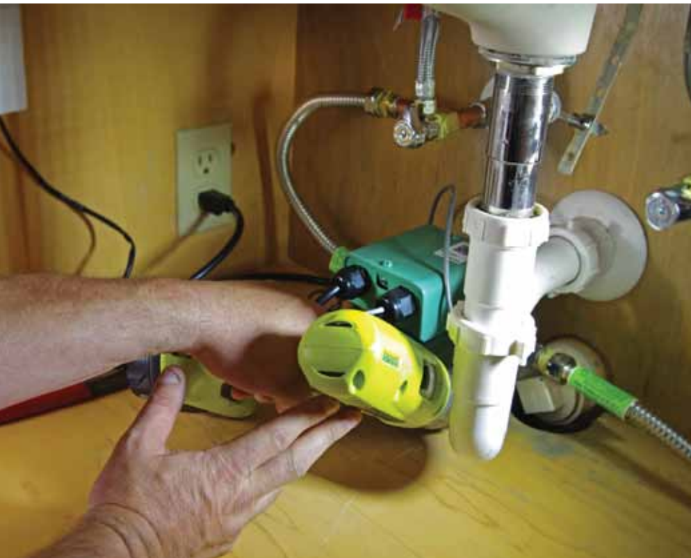
Installation of a hot water recirculation system helped homeowner Kim Ireland save water.
