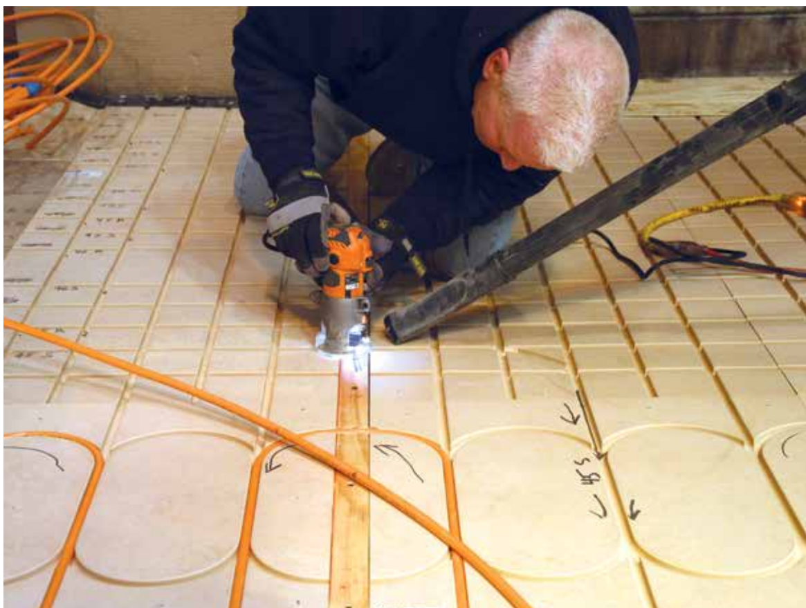
CUT TO SIZE: A Farina Corp. technician uses a router to cut a channel for the PERT tubing. At roughly 10 gallons per minute per manifold, the Watts Radiant system emits 20-35 Btuh per square foot.
