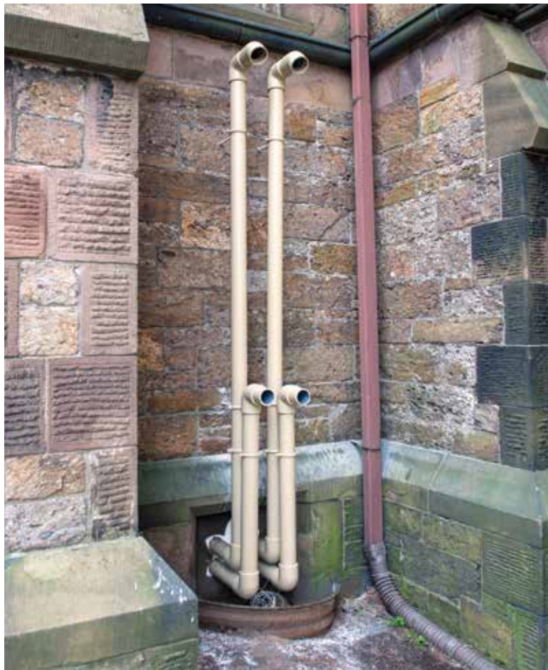
VENTING SOLUTIONS: The design team was challenged with how to vent the boilers in such a huge, solid stone structure.
