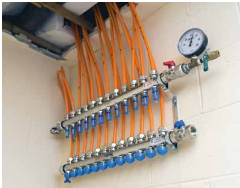
CIRCULATORY SYSTEM: Four large stainless steel manifolds provide circulation to the radiant system below Boston's Church of the Covenant's cavernous sanctuary.
