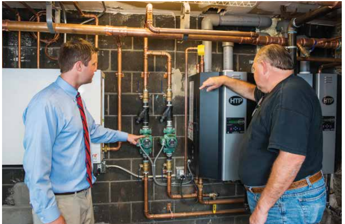
MIXED HYDRONICS: Mike Oppel (left), heating sales, Emerson Swan, and Ray Gircys (right), hang a pre-manufactured Watts radiant Hydronex Panel in the church's basement.
