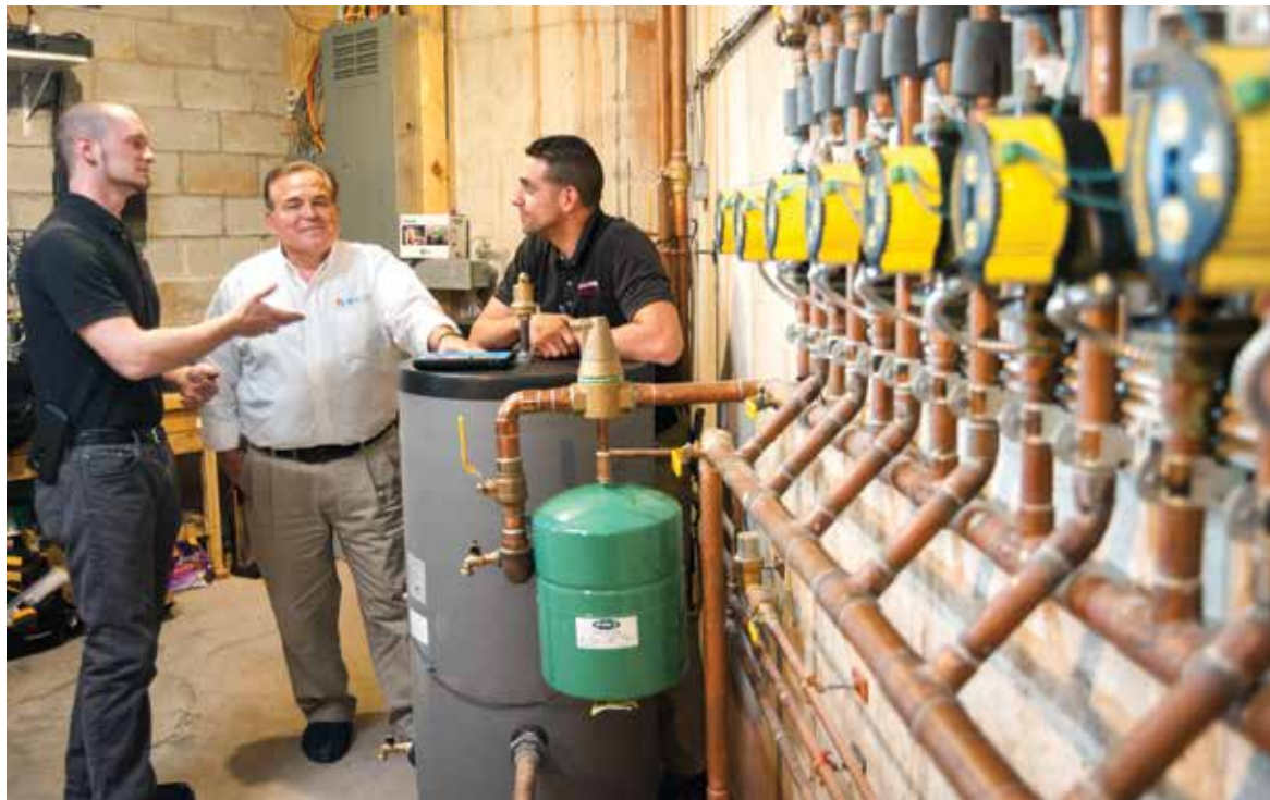
PROFESSOR AND PUPIL: Travis Beveridge (left), Avanti plumber; Anthony Reikow (center), education and training specialist, B.J. Terroni Co.; and Tosco problem solve on location.
