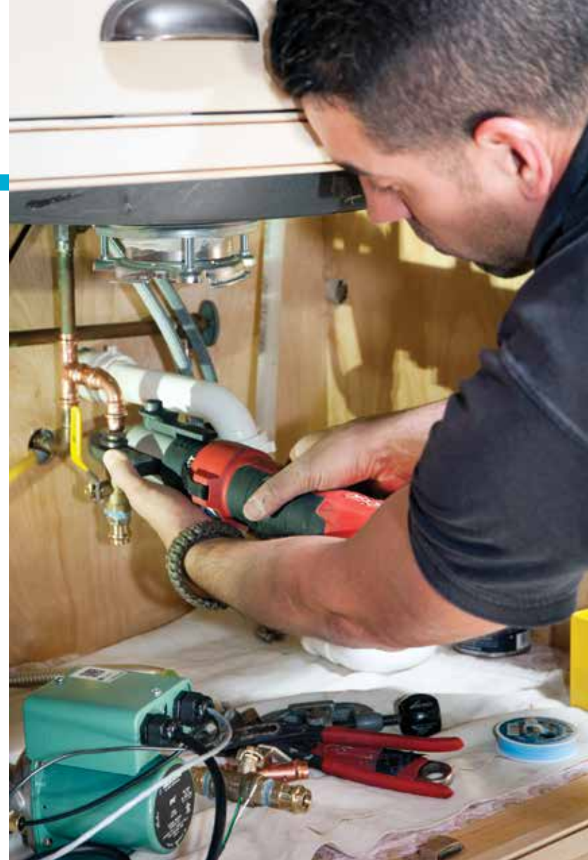
PRECISION PRESSING: Tosco presses a pair of tees under the kitchen sink at a remodeled farmhouse in rural Pennsylvania.
