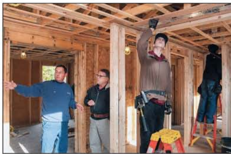
The team of Jim Godbout Plumbing, Heating & Air Conditioning hard at work.
