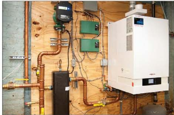
"Five inspectors came through the building and were all astonished by the quality of work in the mechanical room," says Davi Mueller.
