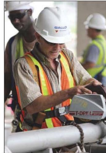
Lightweight stainless steel drainage is easily cut on site during construction of a prison in New Orleans.
