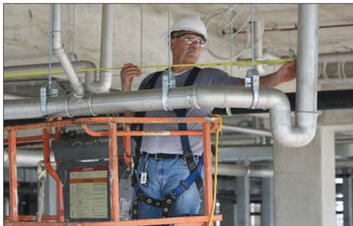
A pipefitter completes a Blücher stainless steel drainage for a large-scale commercial kitchen that serves a prison in New Orleans.
