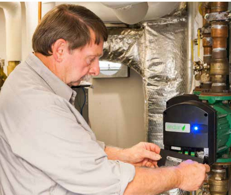
Dan Daley, lead technician at AE Mechanical, in the building's mechanical room.
