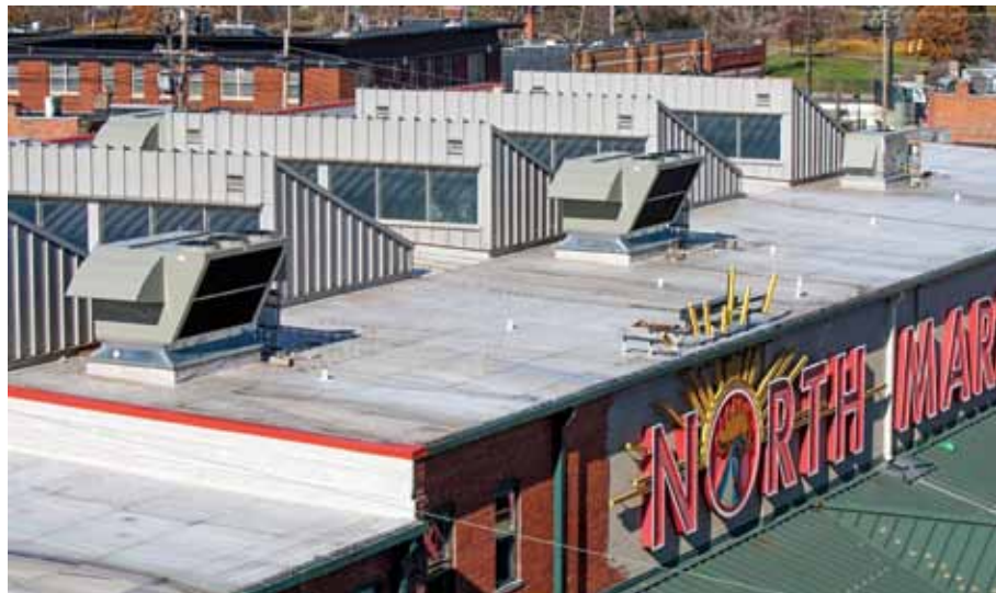
Market roof with air handlers
