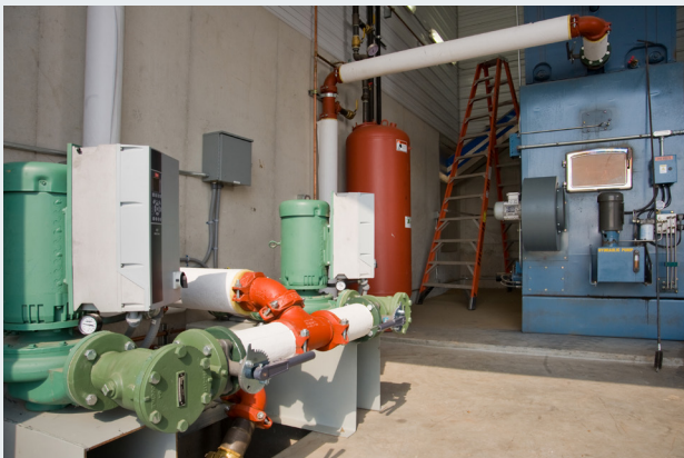
A manure-burning heating system fits well with the overall sustainability theme of Earl Ray Zimmerman’s organic farm. Three-inch water lines run underground to supply both poultry houses with a maximum of 600 MBH each.
