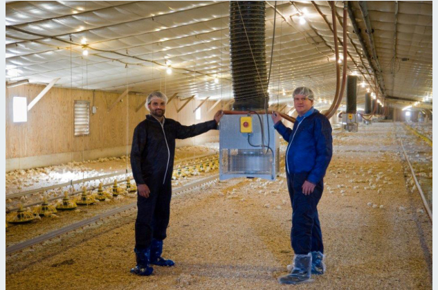
Matthew J. Aungst (left) and John M. Albright, owners of Total Energy Solutions LLC, designed the hydronic biofuel system serving two poultry houses at Earl Ray Zimmerman’s farm.
