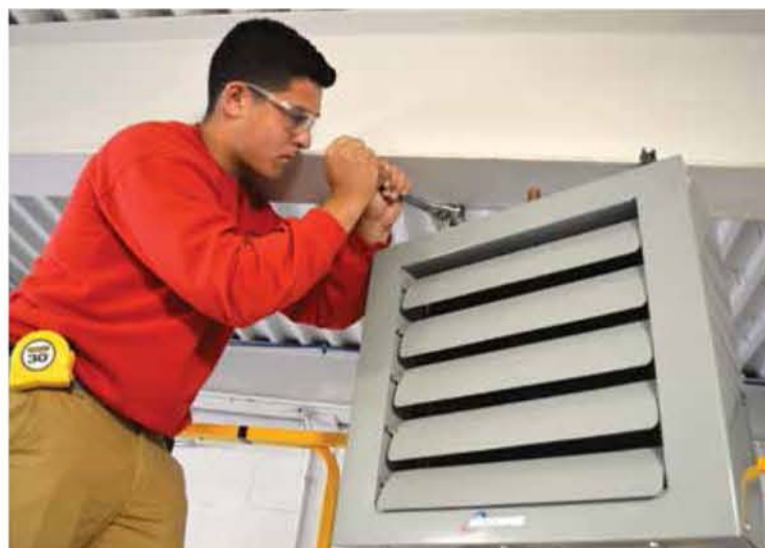
Ekram Rizvani, a senior at Kaynor Tech, secures beam clamps to a Modine unit heater in the garage.
