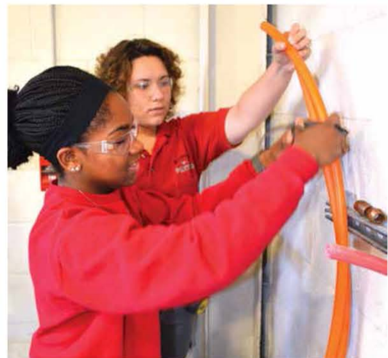
Sydney Craig (foreground) and Erika Hall (background) cut and secure Watts R-Flex in order to prepare the pipe ends for a transition to copper.
