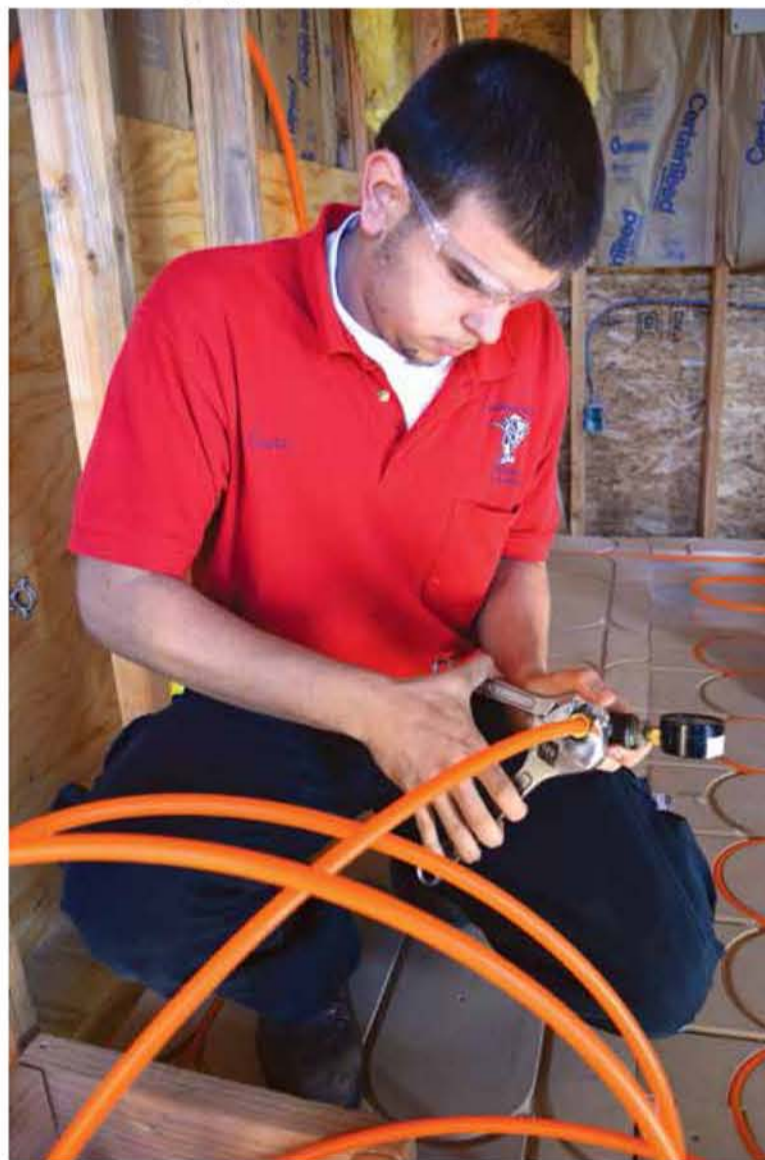
Cesar Quental prepares a pressure test for the Watts Radiant PEX. This will be charged throughout the construction to ensure no leaks occur.
