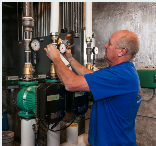
Mike Husmann, co-owner of Husmann Plumbing and Heating, installs insulation on secondary piping connected to a Taco VR15 Viridian pump at Sierra Grande School.
