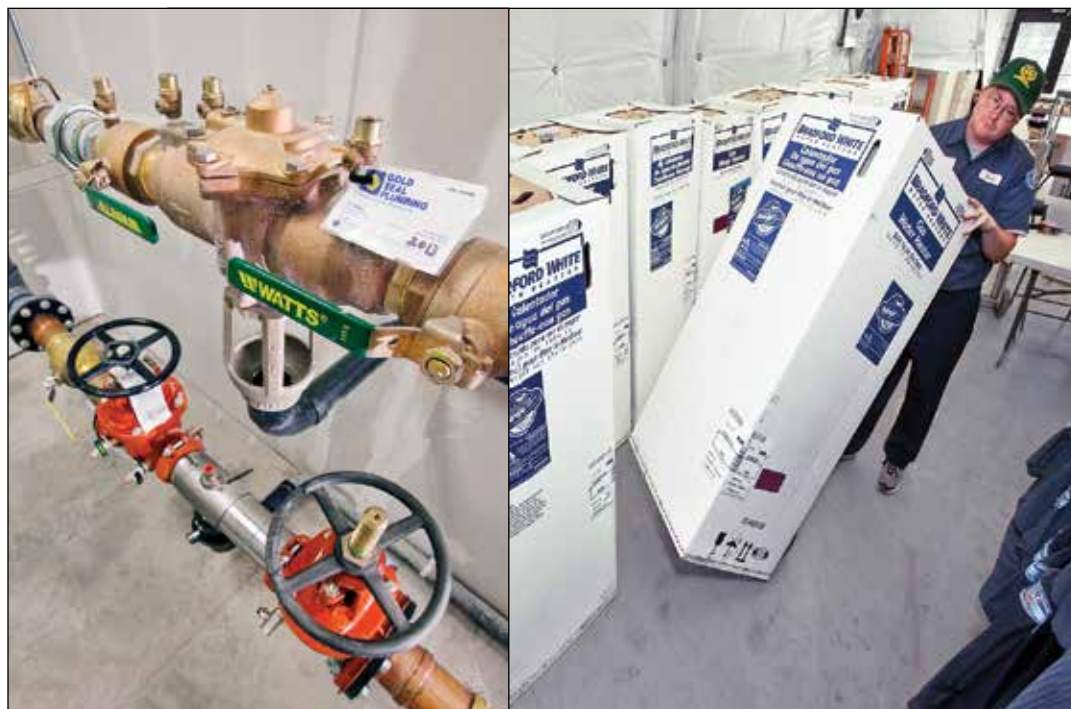
At left, Watts valves and backflow assembly protect domestic water at Affinity at Coeur d'Alene. Right: Gold Seal Purchasing Agent Kevin Peacock pulls a Bradford White water heater out of the warehouse to replace one that had been installed. All of the Gold Seal service vans carry one Bradford White electric and natural gas water heater at all times.
