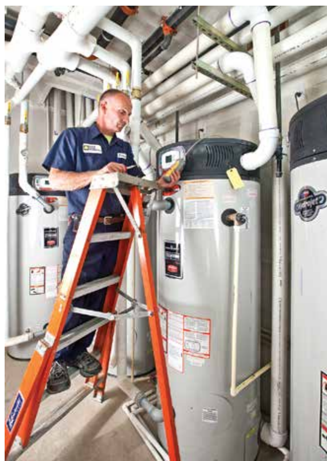
Brian Stanger makes sure the gas pressure is staying constant during a startup check at Affinity at Coeur d'Alene.
