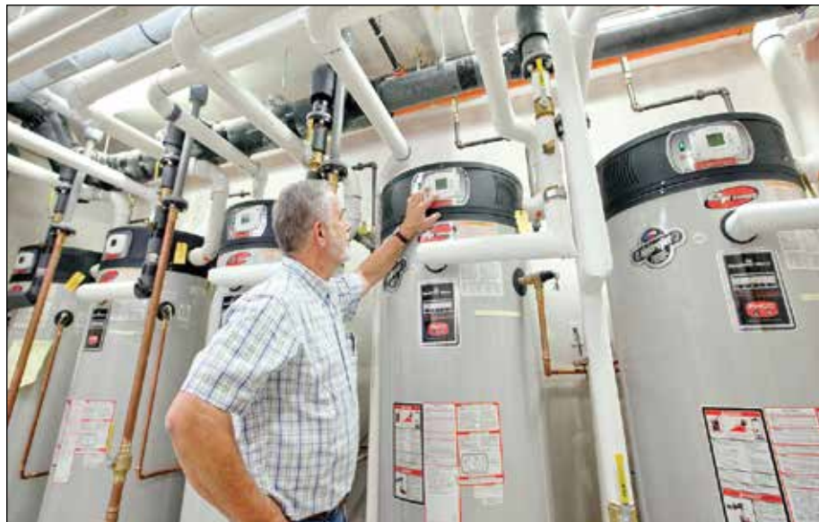
Washington State Bradford White Rep Ron Williams checks the settings of the water heaters at Affinity at Coeur d’Alene.
