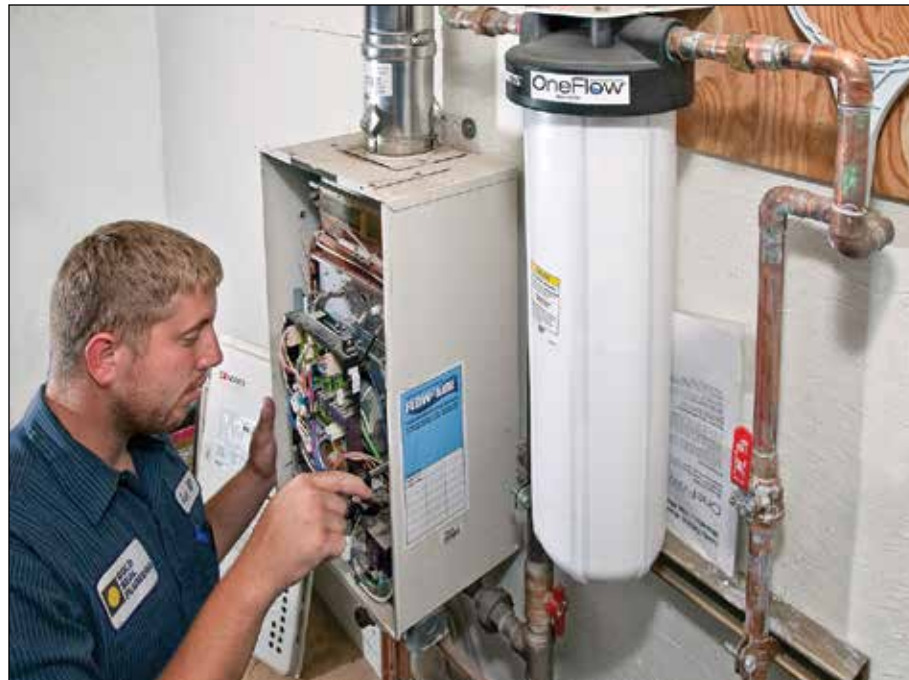
Eric Willis, apprentice at Gold Seal, examines a tankless water heater and Watts OneFlow descaler. Gold Seal has found the water treatment systems to be especially useful at solving vexing water scale problems with heat exchangers.
