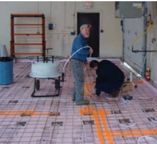
David Palmer, technician (left), and Dan Field (no longer w/the company) install radiant tubing.
