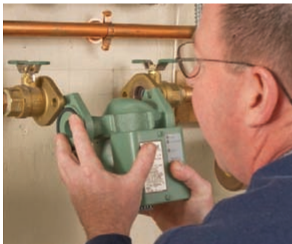
Harry Grattage, foreman, installs a Taco variable delta T pump in a customer’s home.
