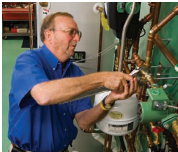
Riley installs a Taco iSeries mixing valve for radiant floor heating at his 2,400-sq.-ft. shop in Warwick, R.I.
