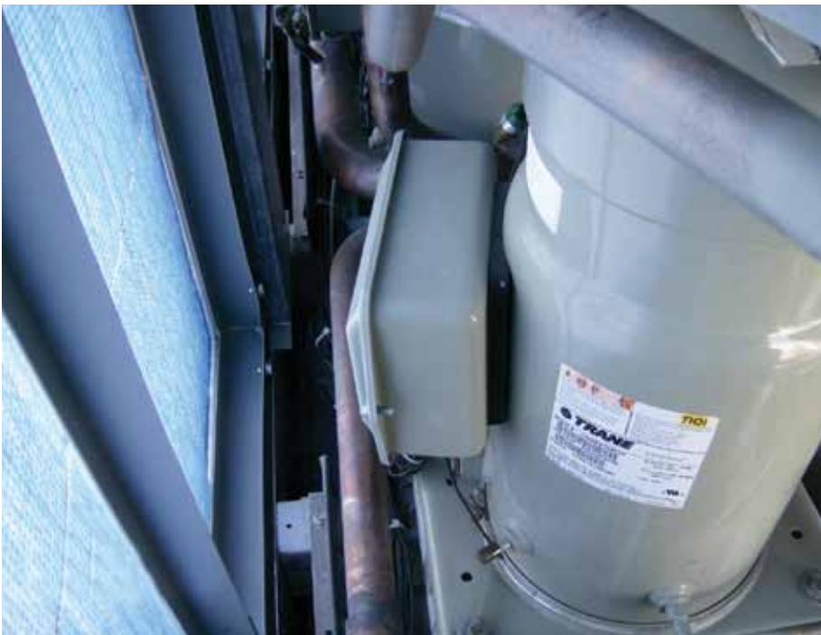
The harvested rainwater is filtered for debris and disinfected with UV treatment before being delivered to spray nozzles that distribute it to the air conditioning condenser coils.
