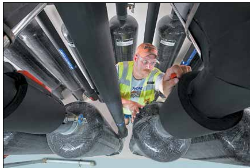
A technician installs a water-processing system using Watts Water Technologies products at Fort Sill, Oklahoma.
