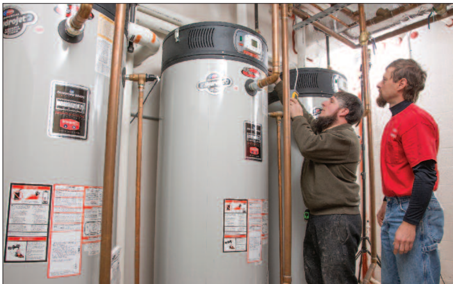
Alan Hershberger, project foreman, left, and Joe Hochstetler, owner of Berlin Plumbing, right, test gas supply pressure for one of the Bradford White eF water heaters.
