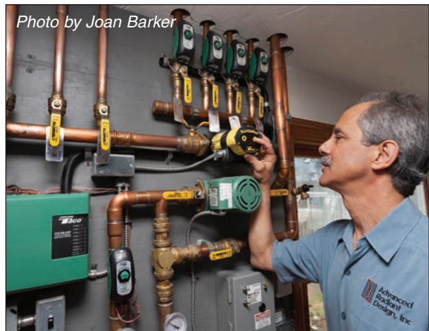
John Abularrage checks the function of a Taco Bumble Bee circulator at another biofuel job just a few miles down the road from the Triform facility.
