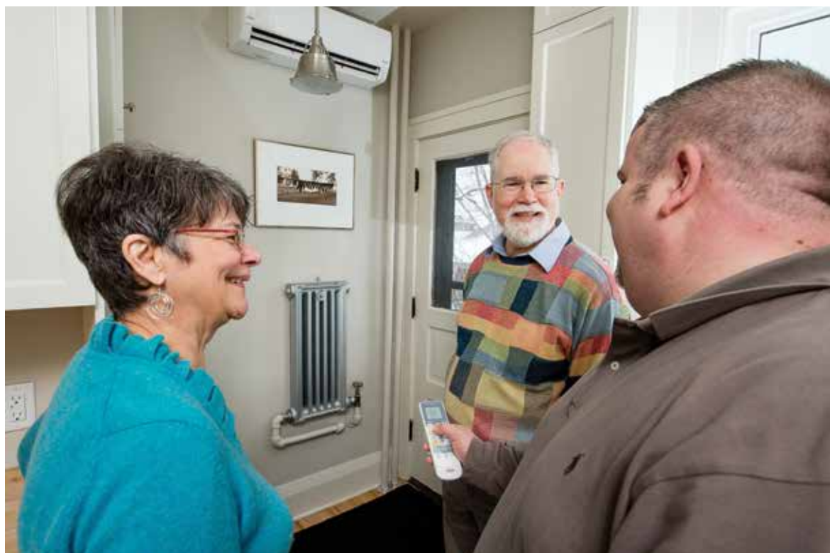
Nick Steckahn, president, Aabott Ferraro (right), introduces Nancy and Bill Rouser to one of the wireless remotes on their newly installed heating and cooling system.
