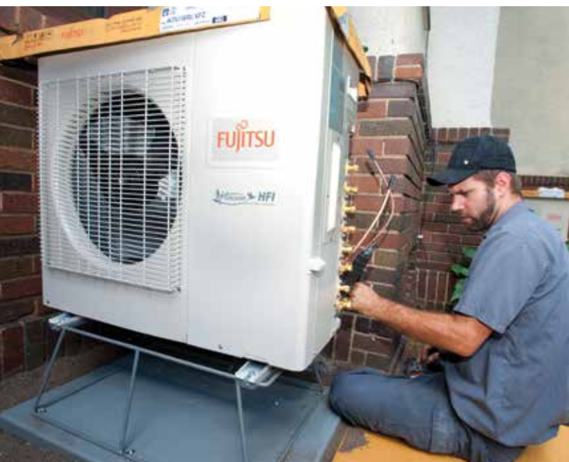
Andert makes a flare connection on the Rouser’s Fujitsu multi-zone condensing unit.
