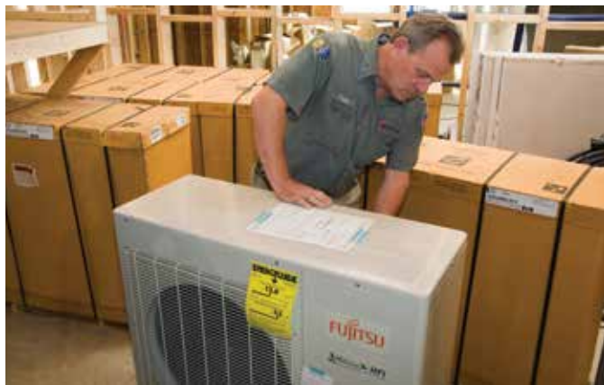
⤴ Frank Simmons, Owner of Simmons Heating and AC, in Hollywood, MD, looks over a unit before installation at the Cornerstone Church.
