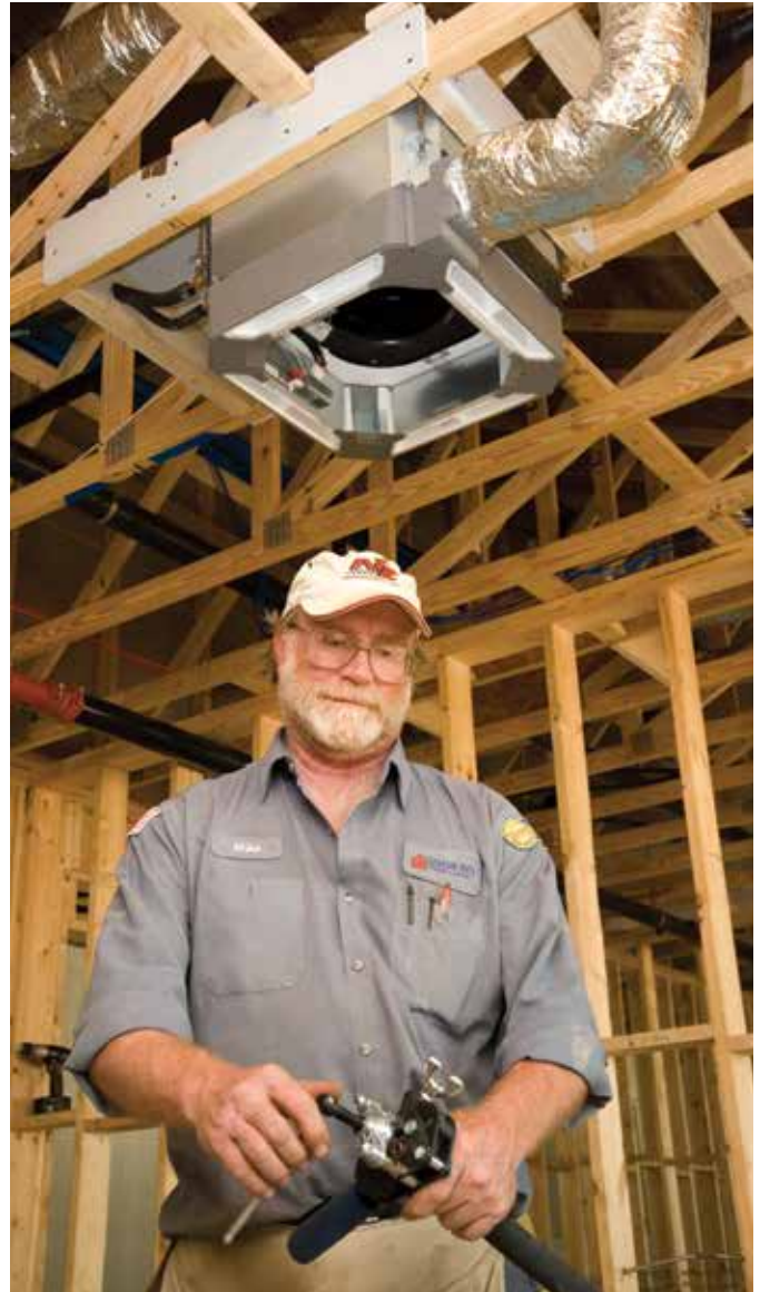
⚡ Mechanic Mike Blaylock prepares a flare fitting for connection to a ceiling cassette unit.
