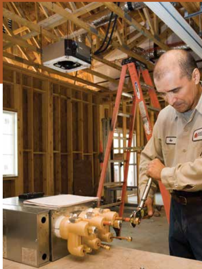
⤴ Jose Cortes, Technician’s Helper, getting ready to put together a distribution box at a Cornerstone church.
