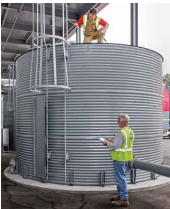
The rainwater harvesting system includes five tanks for a total capacity of 42,000 gal.
