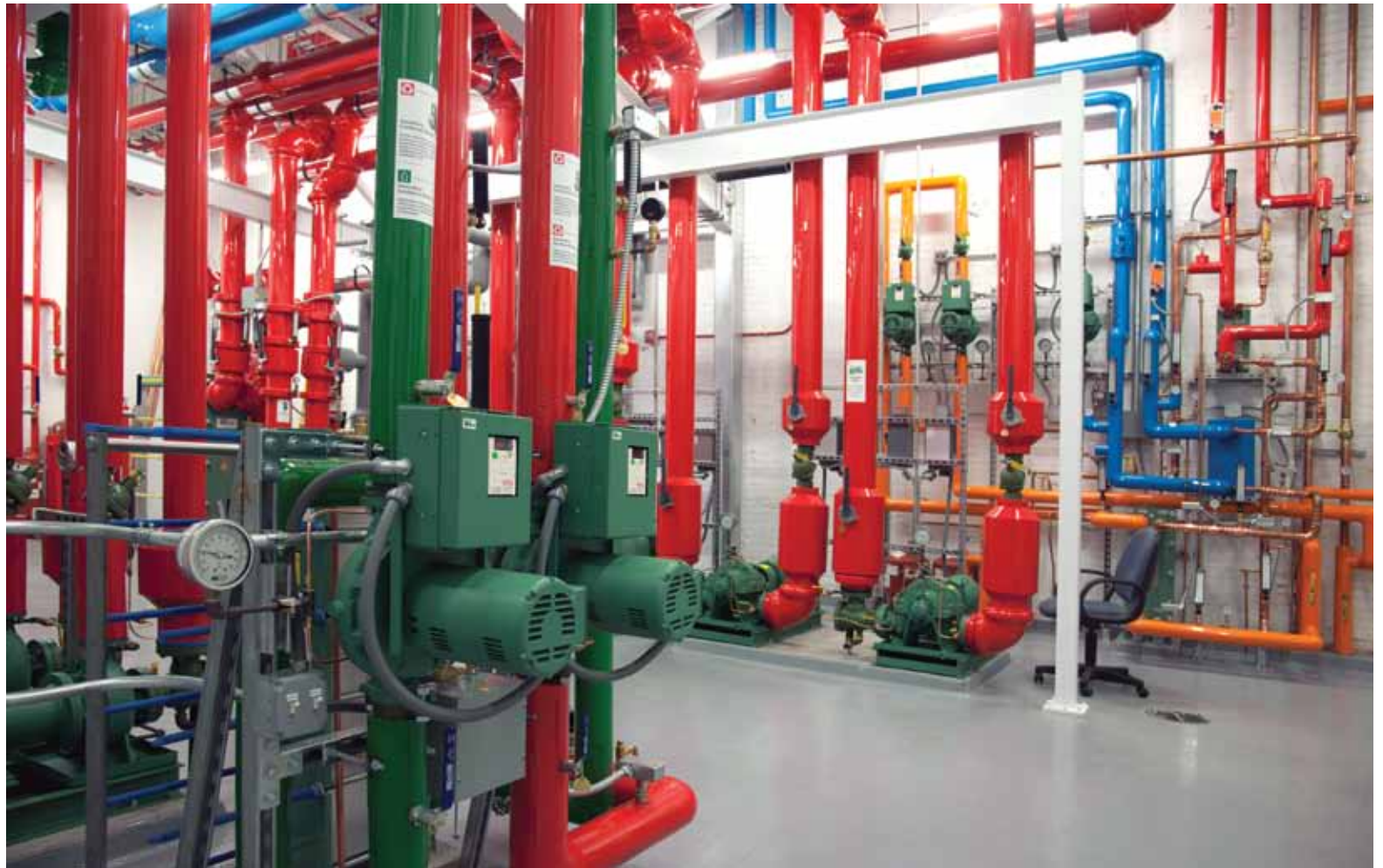
The design and application of hydronic systems, like this one, is being enhanced by innovative smart technology.
