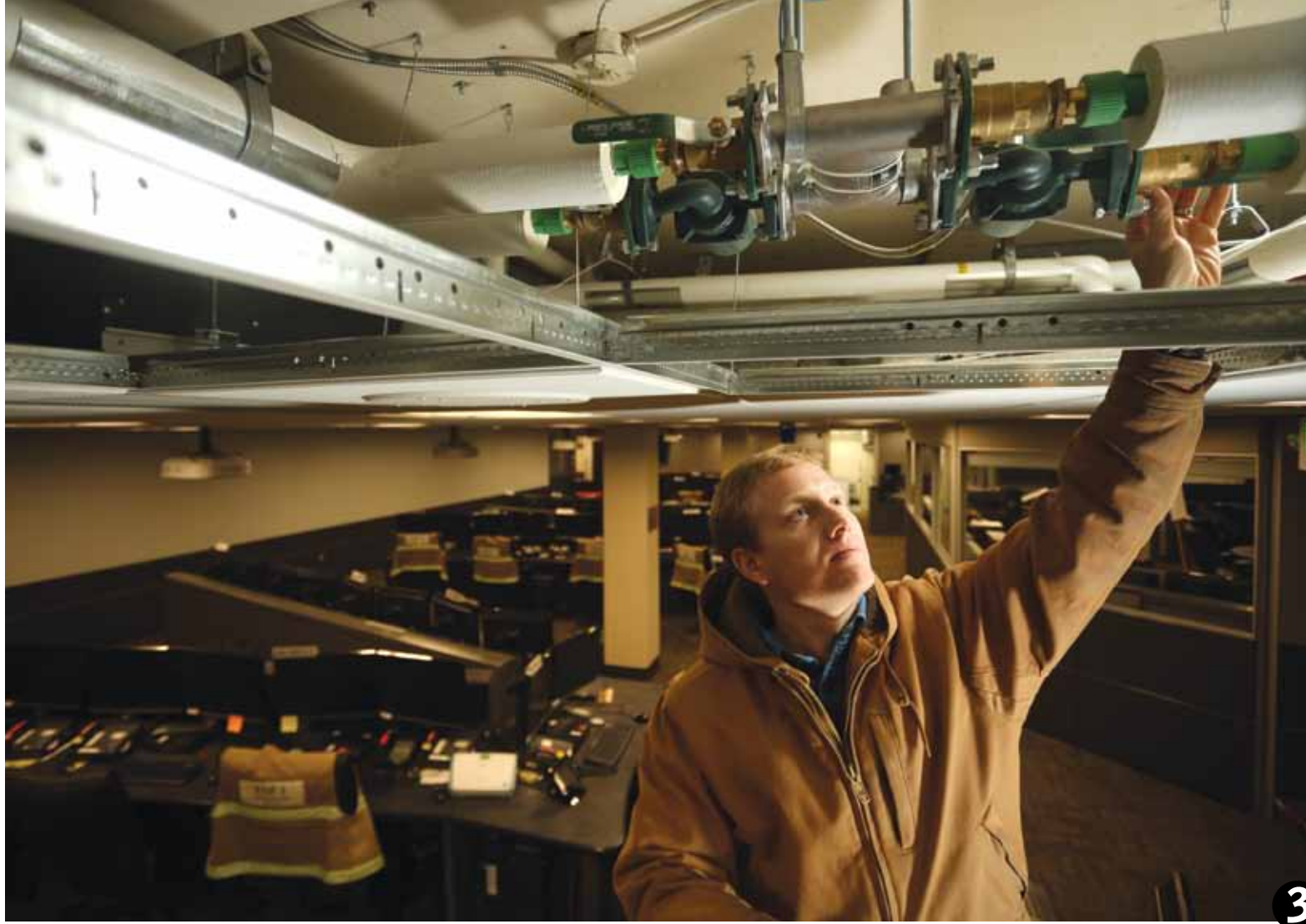
❶ Jeremy Pennington, Mechanical QC, inspects part of the installation at the Emergency Operations Center on Joint Base Elmendorf-Richardson Air Force Base, near Anchorage, Alaska. ❷ Weldin Construction's Mechanical Division installed the hydronic system at the Emergency Operations Center, on base at Joint Base Elmendorf-Richardson. ❸ The chilled beam hydronic installation provides both heating and cooling for the facility.
