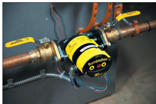
Two Delta-T, ECM Taco BumbleBee circulators work symbiotically with variable-flow manifolds. The benefit of each component multiplies that of the other.
