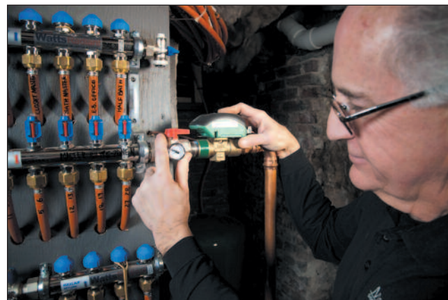
Swatton watches the supply temperature rise on one of the manifolds immediately after a zone valve opens.
