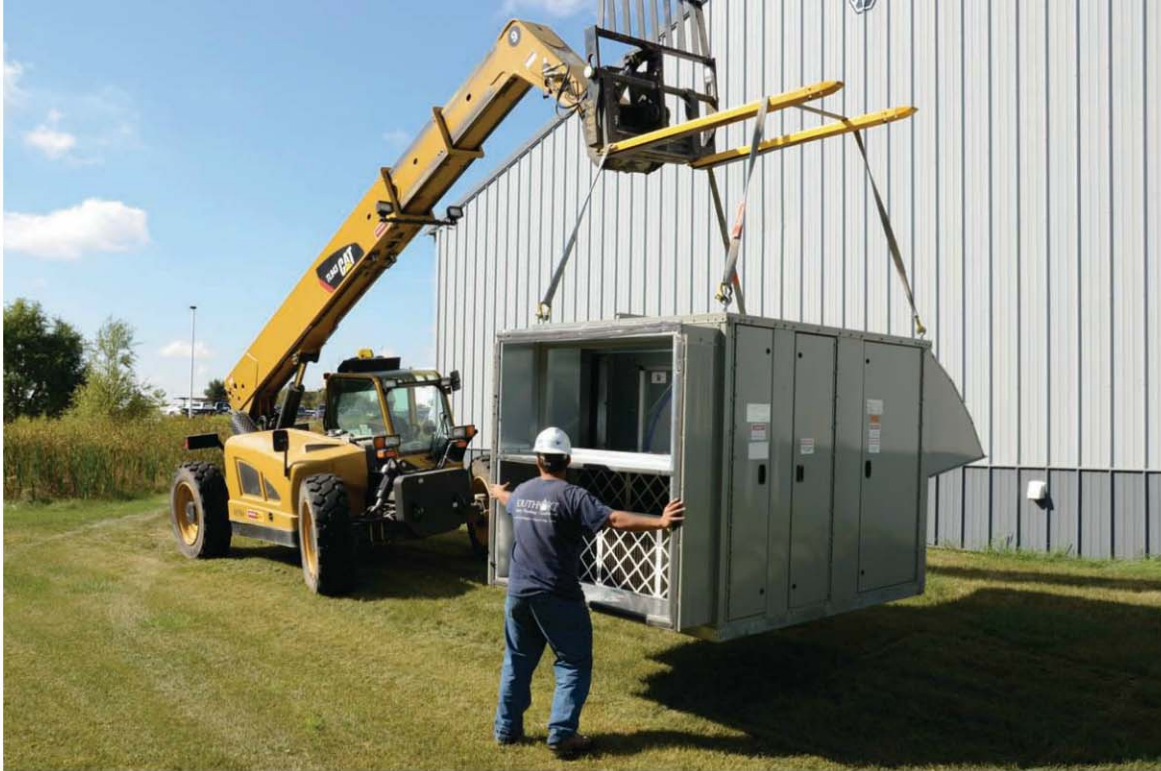
HVAC technician Josh Pothast stabilizes the Atherion's ERV module as it's moved into position.
