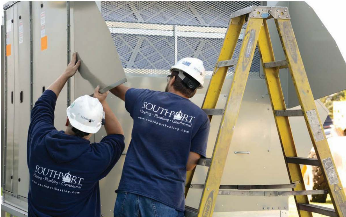
If an existing roof isn't engineered to support the weight of a packaged unit, installing equipment on a frame at ground level is sometimes an option.
