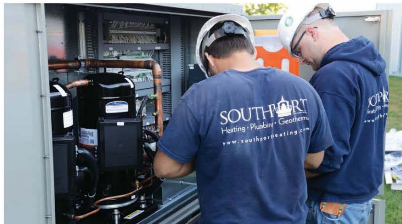
Southport Heating, Plumbing, and Geothermal technicians Josh Pothast (left) and Nicholas Draeger (right) install a 30-ton Modine Atherion rooftop packaged unit at Rite Engineering, in Franksville, Wis. The unit provides heating, cooling, and IAQ with the added benefit of an energy recovery ventilator (ERV).
