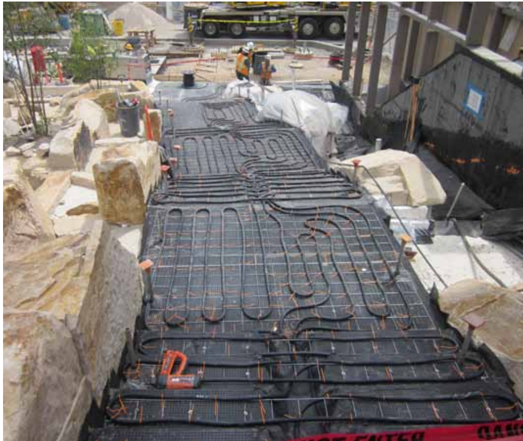
Exterior stairways at City Creek Center receive snow-melting warmth from three-quarter inch Onix tubing, chosen for its superior flexibility.
