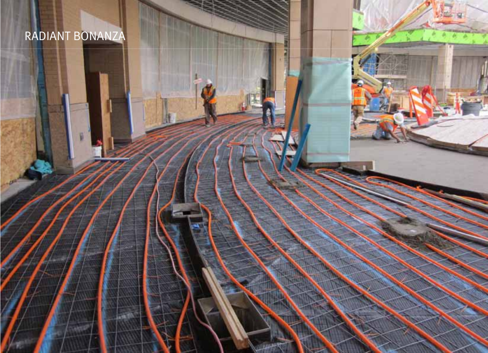
More than 102,000 lineal feet of 5/8" Watts Radiant PEX+ tubing was installed in throughout both of the City Creek Center malls, providing warmth in the winter and cooling in the summer.
