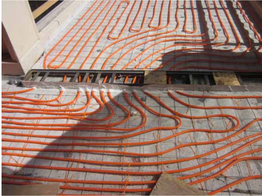
CCI Mechanical supervisor Seth Roth said, "If I never see another zip tie, I won't mind at all" after his crews used the most cautious means of connecting PEX tubing to rewire in the upper levels of the malls at City Creek Center.
