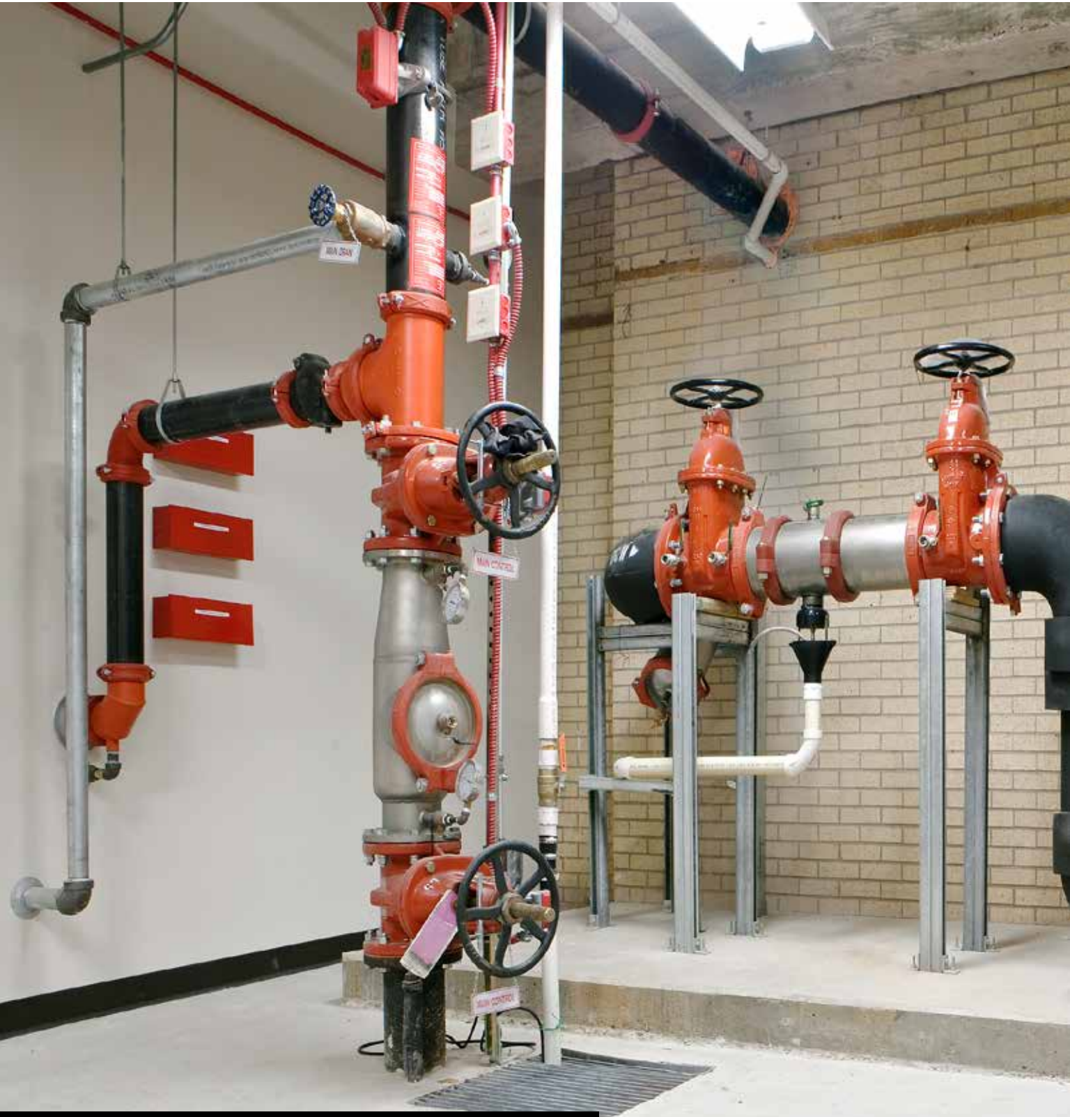
Four and eight-inch Watts model 957 RPZ backflow preventers protect the domestic water system. Strainers installed upstream of the RPZs help keep debris from getting into the OneFlow system and backflow preventers.
