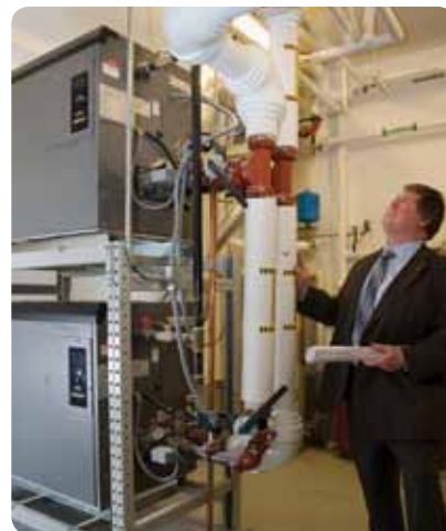
ECI Mechanical Engineer, Don Swick, reviews the boiler installation at Carlos Gilbert Elementary School.
