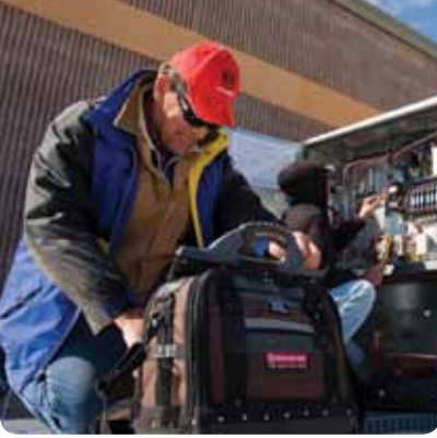
Richard MacDonald, ECI service technician, performs scheduled maintenance for an Aaon roof top unit at Aspen school.
