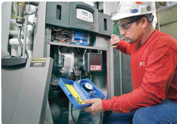
Venting should be checked annually. Using the proper test equipment is one way to ensure that there's no blockage of sealed-combustion systems exhaust, such as that found on this Laars NeoTherm boiler.
