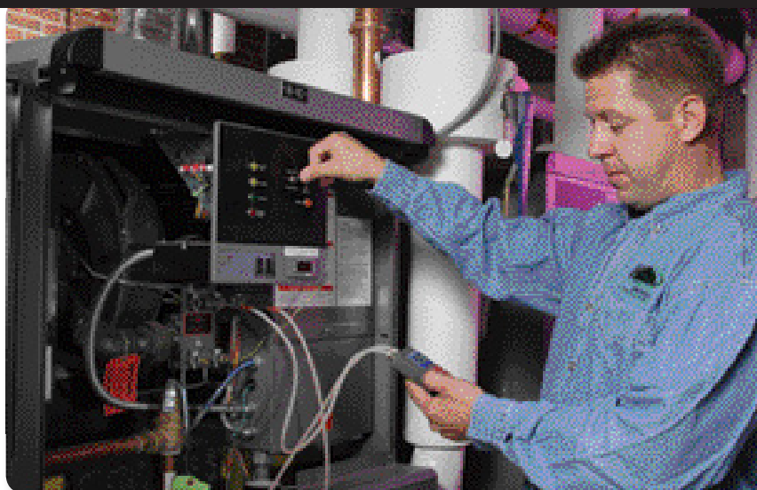
Routine maintenance of boilers such as this Laars Rheos includes CO 2 testing. If adjustments are required, the use of test equipment verifies proper gas/fuel mixture, an important step for sealed-combustion or modulating/condensing appliances.
