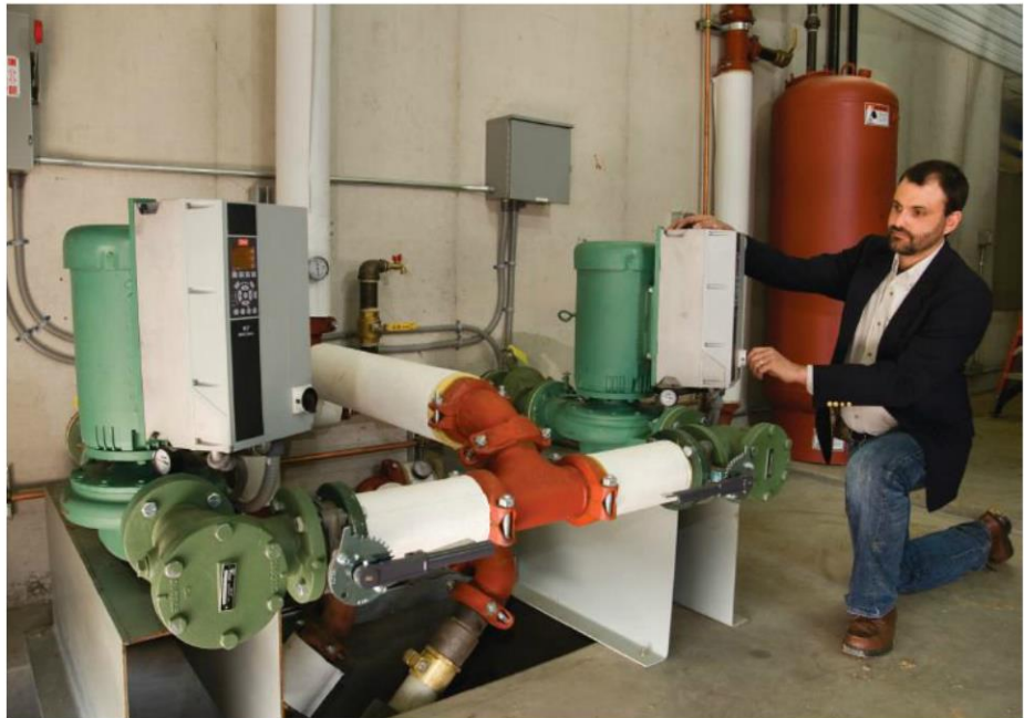
Matt Aungst , who designed the distribution portion of the project, tests redundancy of the system's two pumps. Pump A runs as "duty," leaving Pump B for backup. After 84 hours of runtime, the pumps automatically switch roles.
