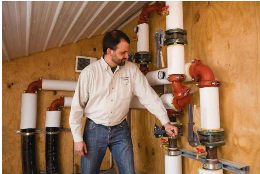
Aungst stands in a manifold room between the two chicken houses. There are no secondary pumps or pressure sensors anywhere in the system. The pumps in the mechanical room sense even the most minute pressure changes anywhere in the system.
