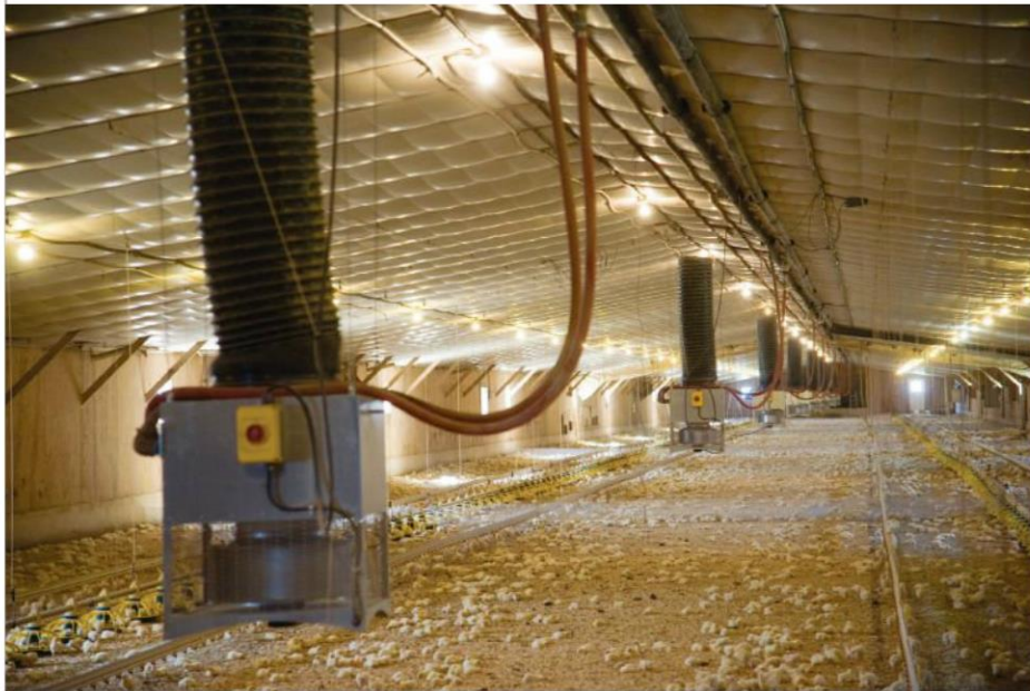
The advanced hydronic biofuel heating system conditions two 500-ft. chicken houses. Each building contains up to 30,000 birds, which grow from peep to slaughter weight in roughly six weeks.
